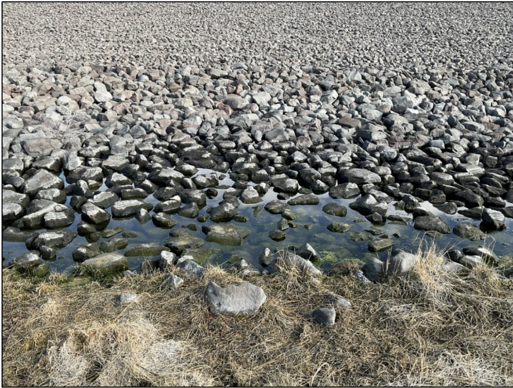
PL-7. Ponding Water on South Disposal Cell Apron
