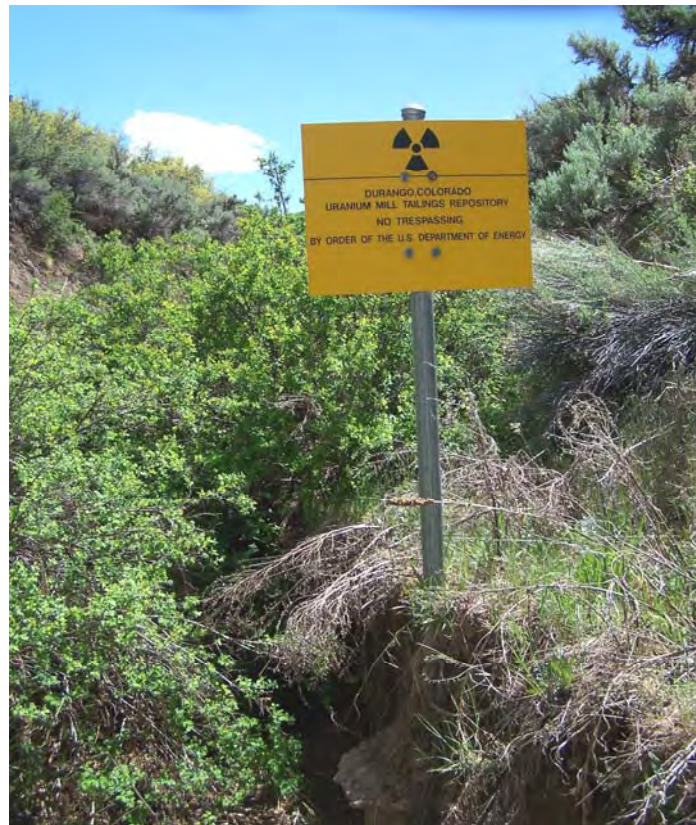
DUR 5/2008. PL-2. Undercutting at perimeter sign P44.
