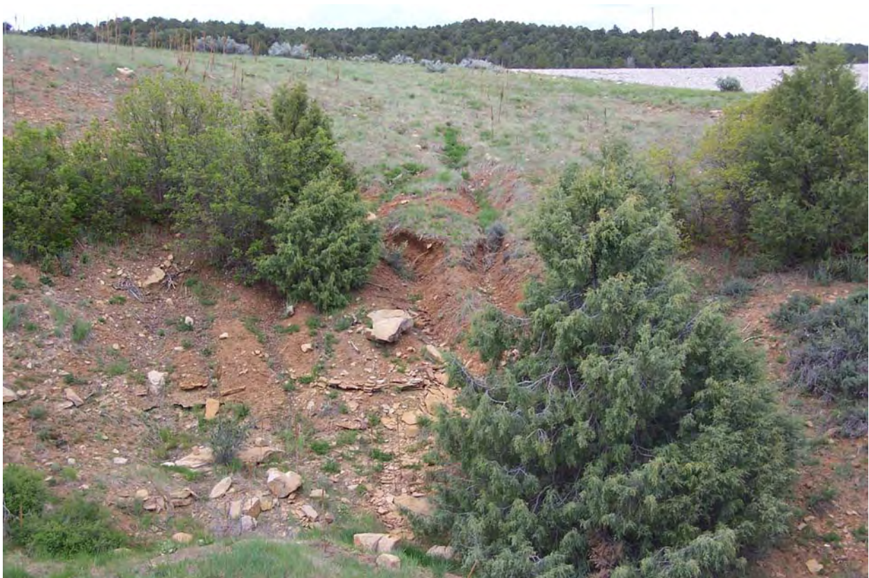
DUR 5/2008. PL-4. Headcuts of gullies below southwest corner of disposal cell.
