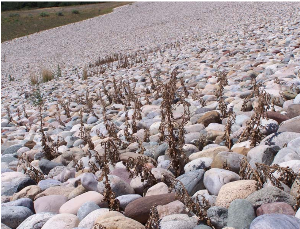
DUR 8/07. PL-4. Dead Canada thistle on disposal cell side slope, sprayed with herbicide in June 2007.
