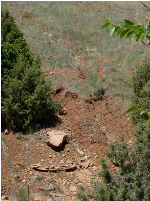
DUR 6/2010. PL-3. Headcuts of gullies below SW corner of disposal cell; no change from 2009
