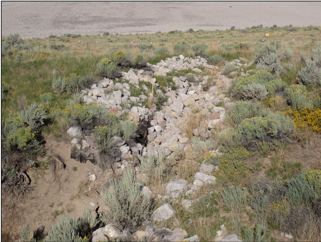
PL-9. Exposed Geofabric in Swale No. 2
