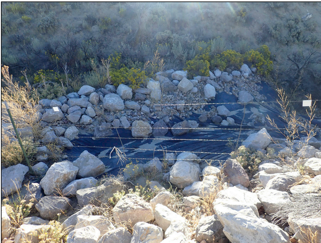
PL-8. Exposed Geofabric in Outlet of Swale No. 1
