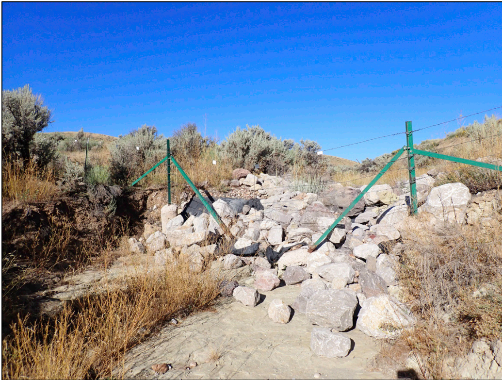
PL-7. Exposed Geofabric Below Diversion Channel No. 1
