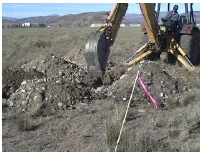
Figure 4-8. Excavation on the Millsite in November 1999 (View 4) Note: Excavated material was separated in different piles and backfilled in the same order
