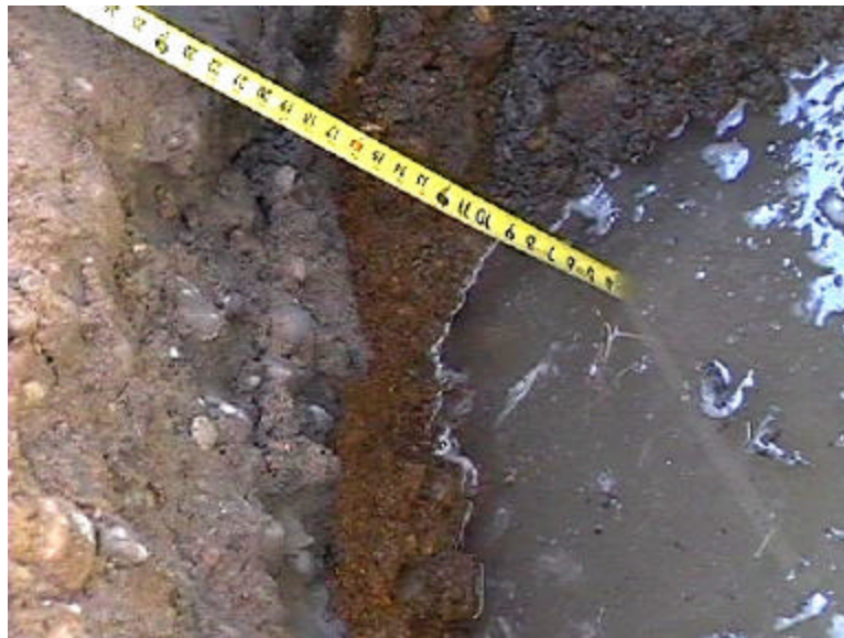
Figure 4-14. Rusty Colored Sediment at Location 544
