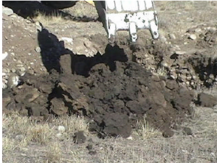
Figure 4-5. Excavation on the Millsite in November 1999 (View 1) - Note: high clay content select fill material
