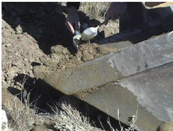
Figure 4-7. Excavation on the Millsite in November 1999 (View 3) Note: Sediment and water samples were taken from the backhoe bucket
