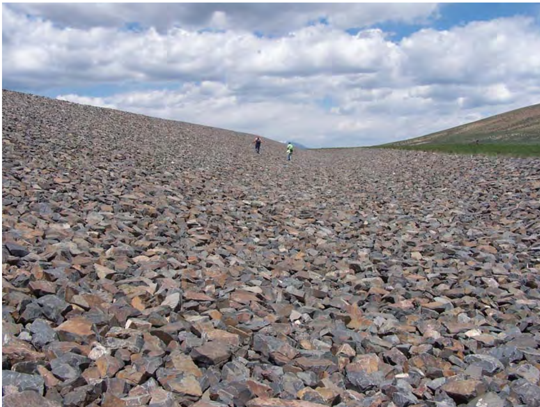
GUN 6/2008. PL-4. East diversion channel along the northeast side of the disposal cell.
