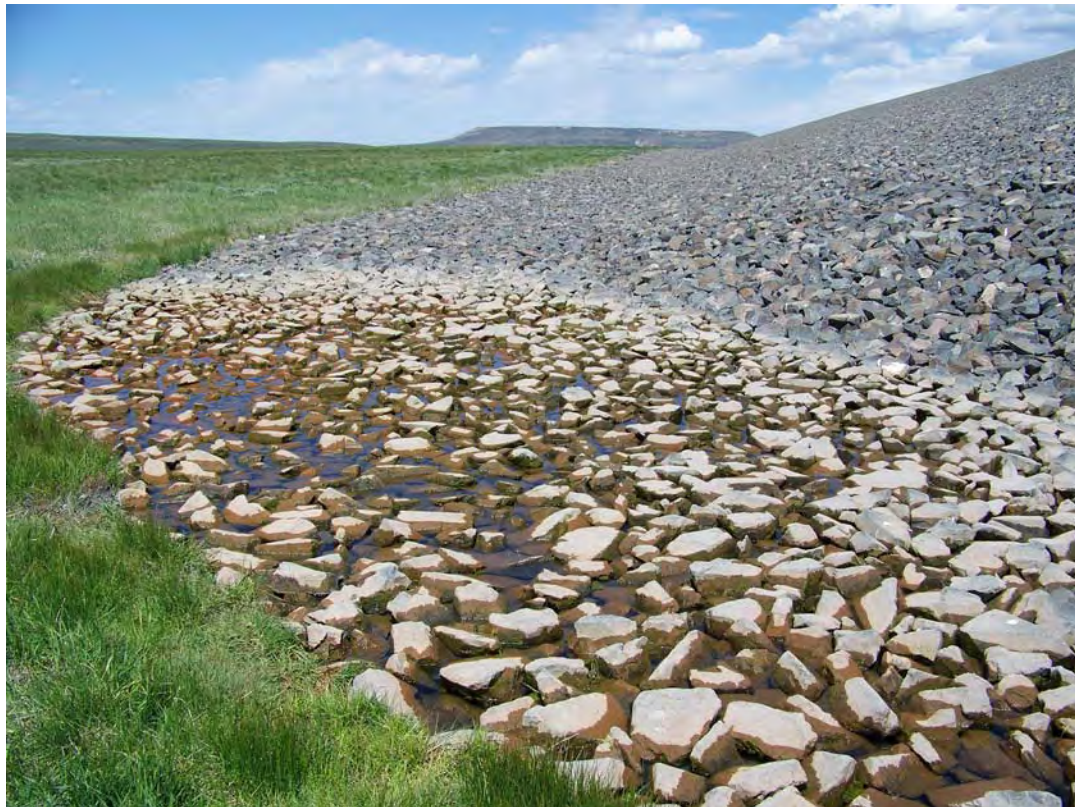
GUN 6/2008. PL-6. Ponded water at the southeast corner of the disposal cell.
