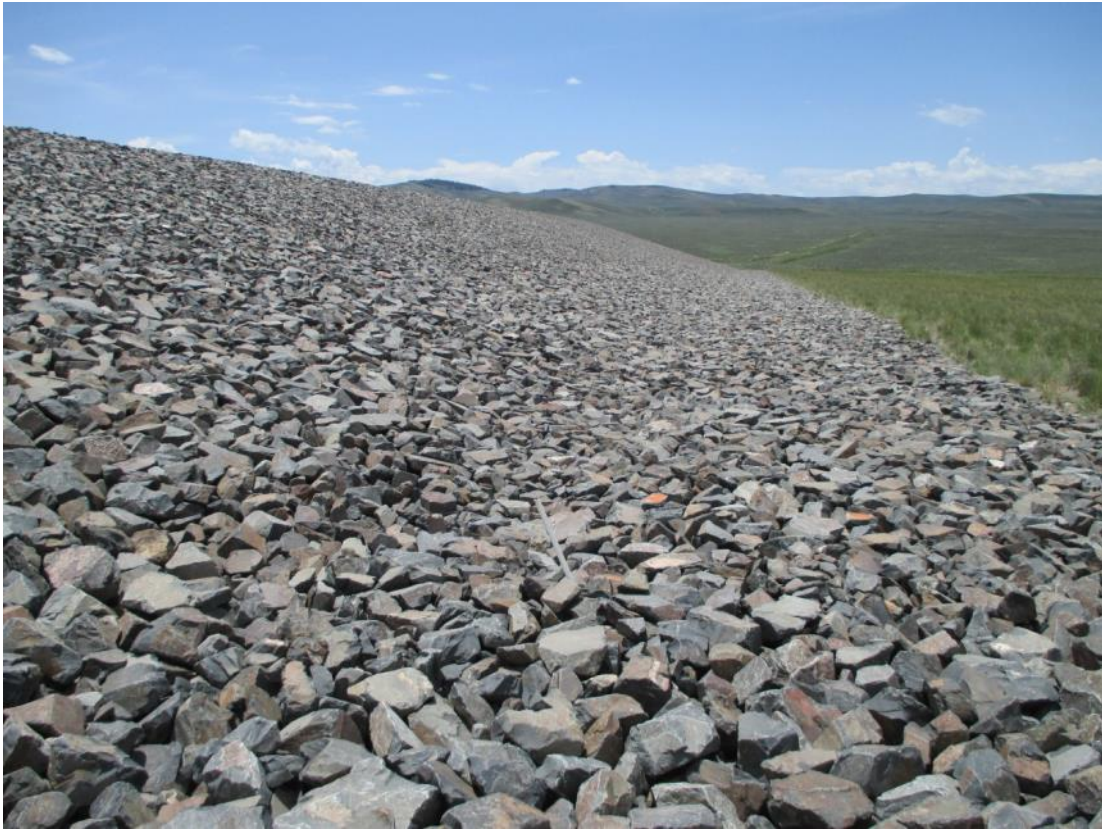
GUD 6/2014. PL-7. West side slope and apron of disposal cell; Riprap Test Area No. 3 in foreground.
