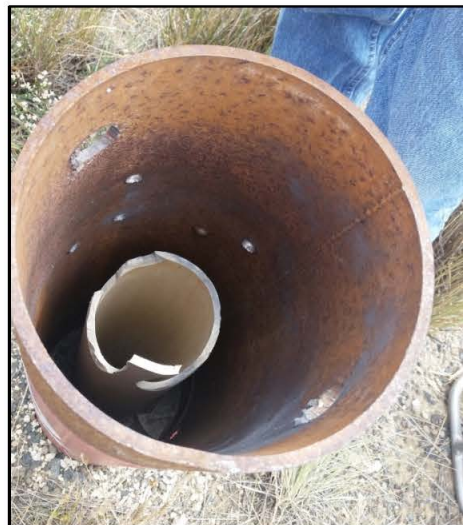
Figure 1. Damaged Riser at Monitoring Well 0712
