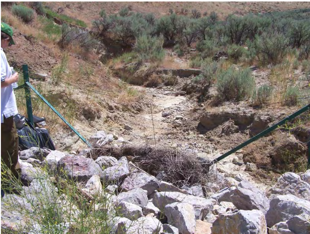
MAY 7/2008. PL-4. Erosion (headcutting) at discharge point of Diversion Channel No. 1.
