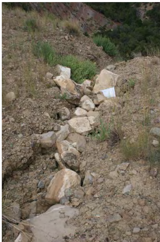
RFL 8/2008. PL-4. Armored gully at the base of the interceptor trench.
