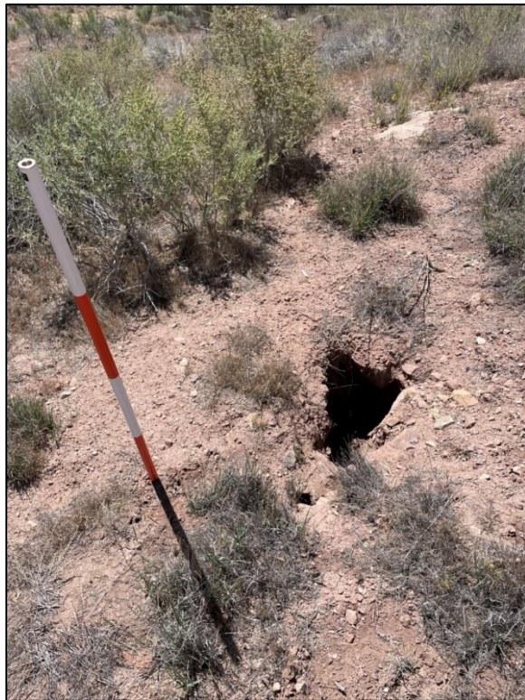
PL-8. Soil Piping West of Access Road
