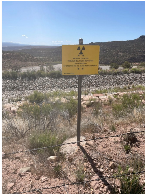
PL-1. Erosion Around Concrete Base of Perimeter Sign P22
