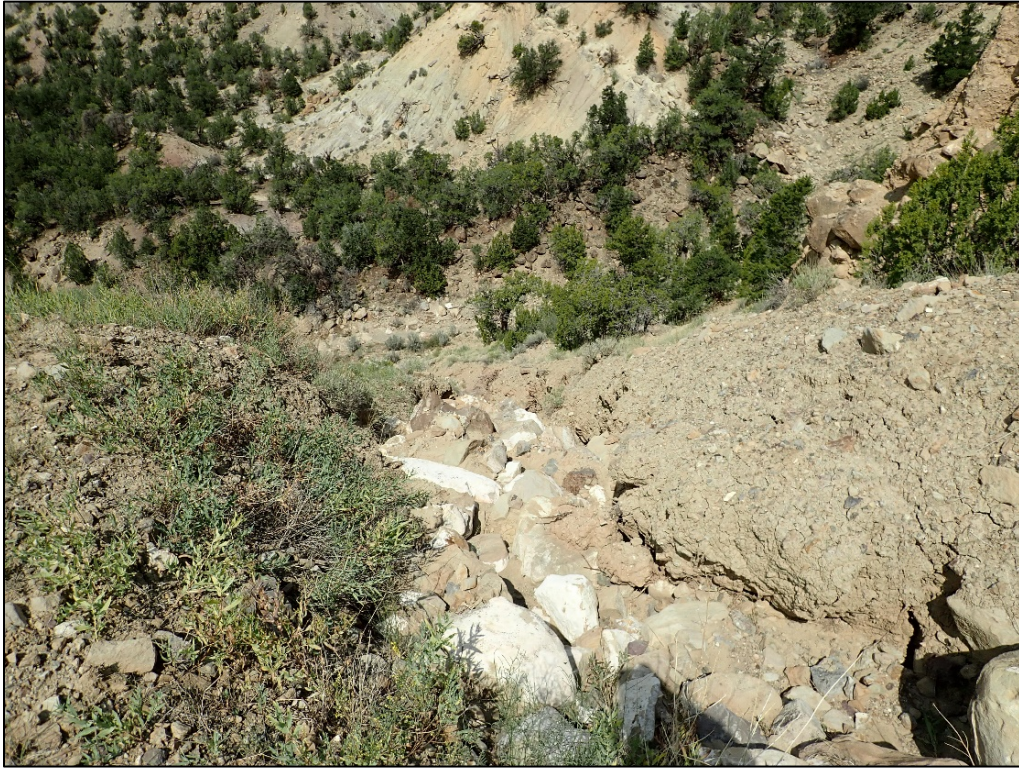
PL-8a. Gully Erosion in Interceptor Trench Outfall in 2021
