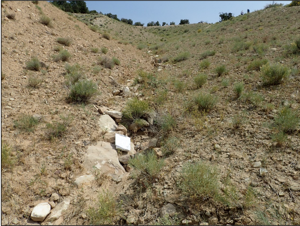
PL-7a. Gully Erosion in Interceptor Trench Outfall in 2021
