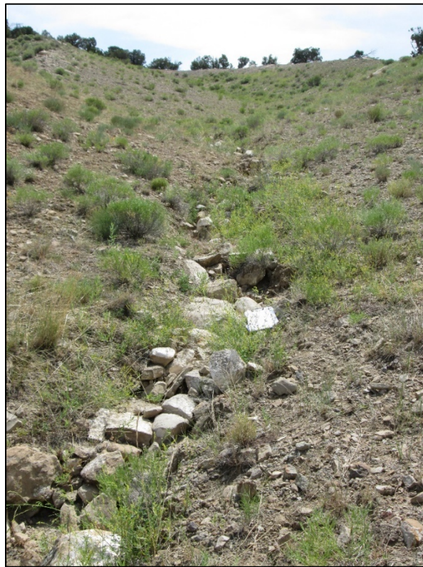
PL-7b. Gully Erosion in Interceptor Trench Outfall in 2016—Photo for Comparison
