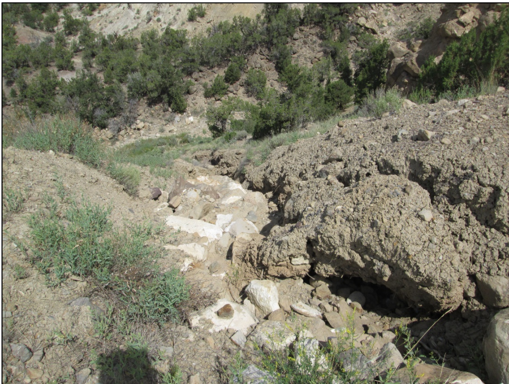
PL-8b. Gully Erosion in Interceptor Trench Outfall in 2016—Photo for Comparison
