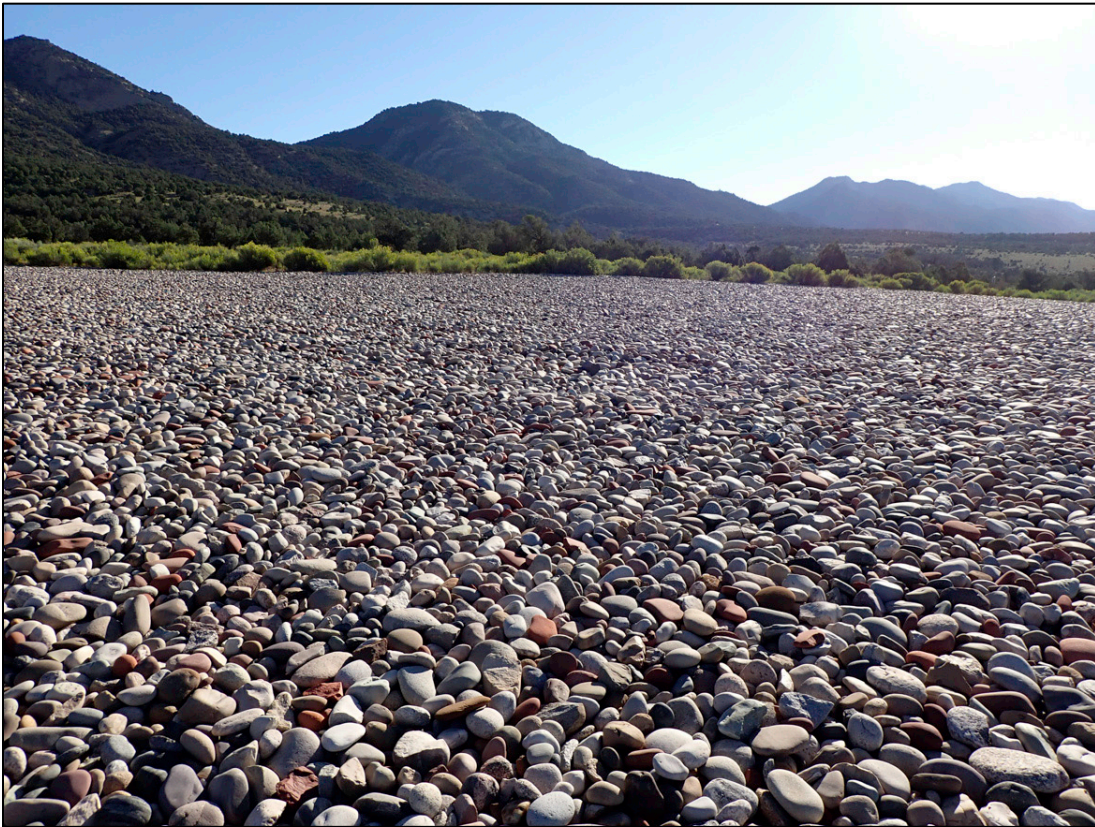
PL-8. Depression on Top Slope in Southeast Area of Disposal Cell
