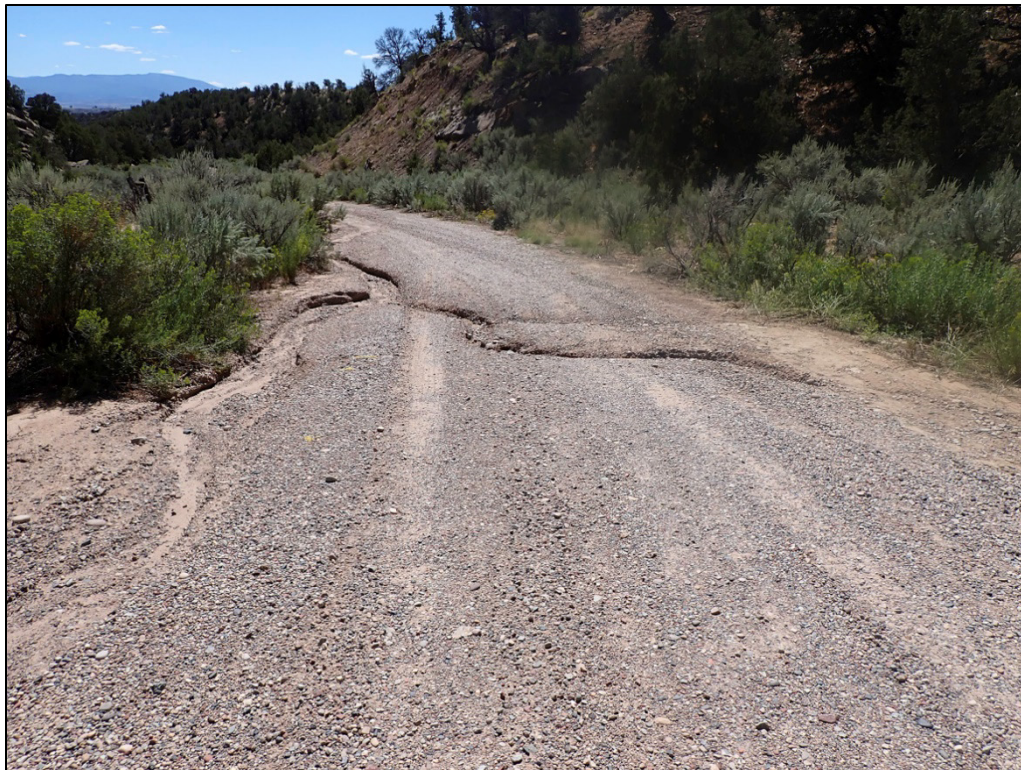
PL-2. Rutting and Erosion Along Access Road
