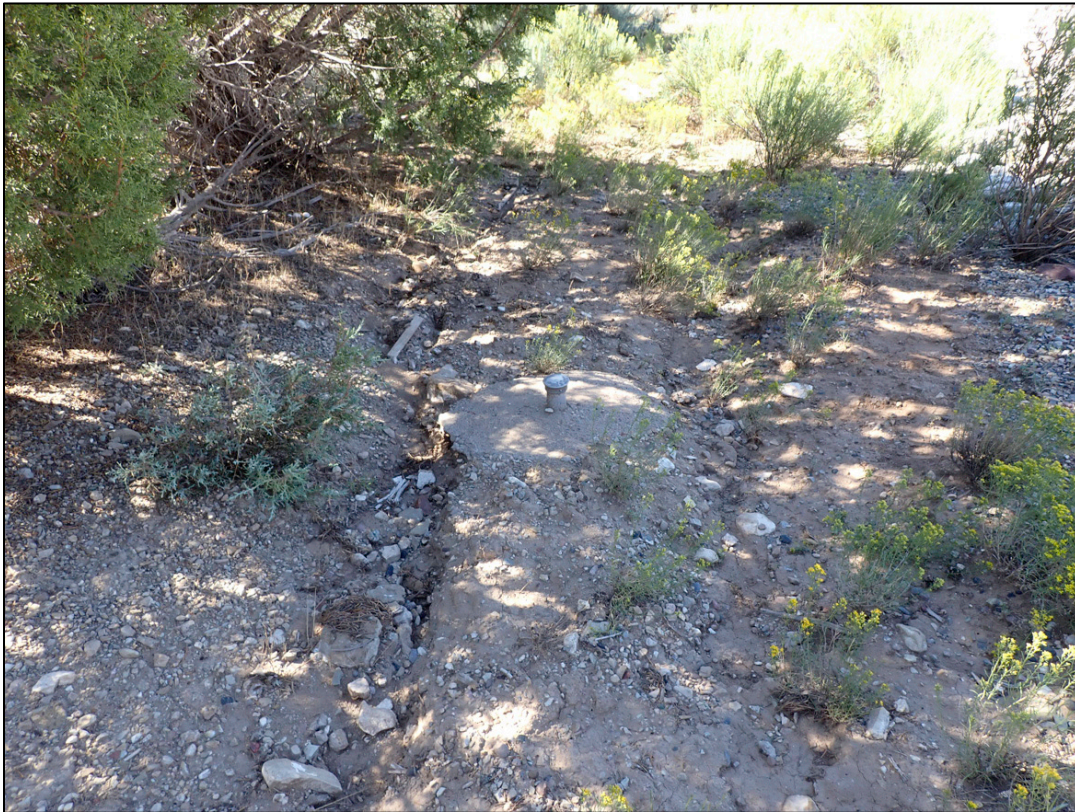
PL-5. Boundary Monument BM-3 with Concrete Base Undercutting
