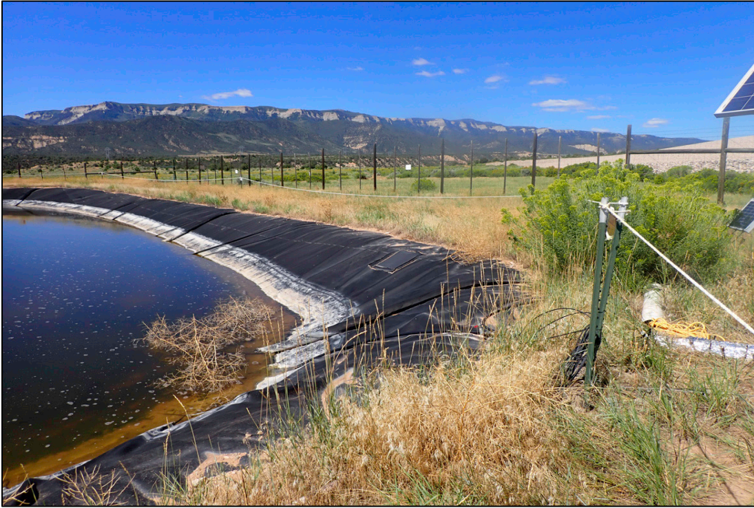
PL-7. Evaporation Pond Liner with Repair Patch on Northern Corner
