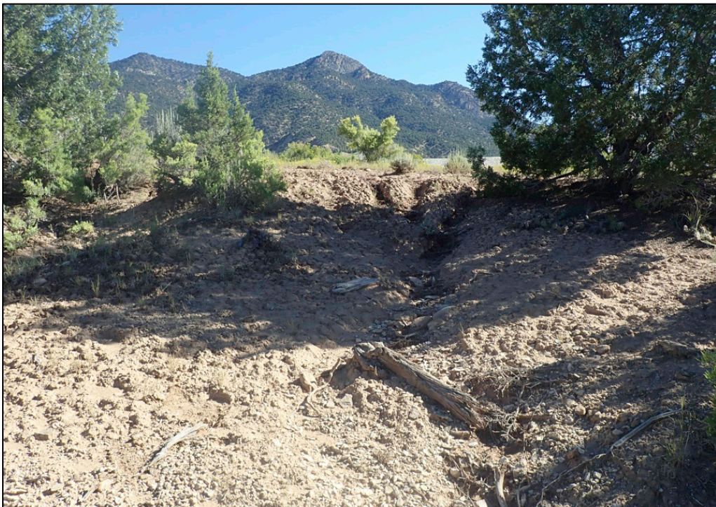
PL-10. Erosion near Perimeter Sign P26
