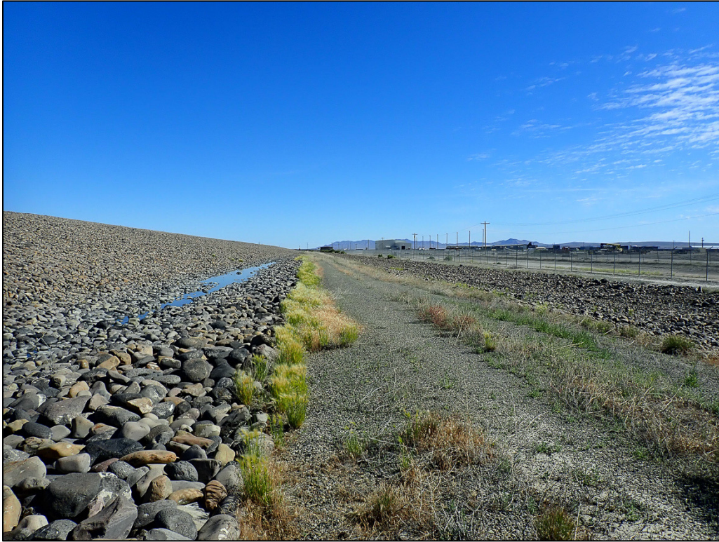
PL-9. Ponded Water in Toe Drain near Southeast Corner of Disposal Cell
