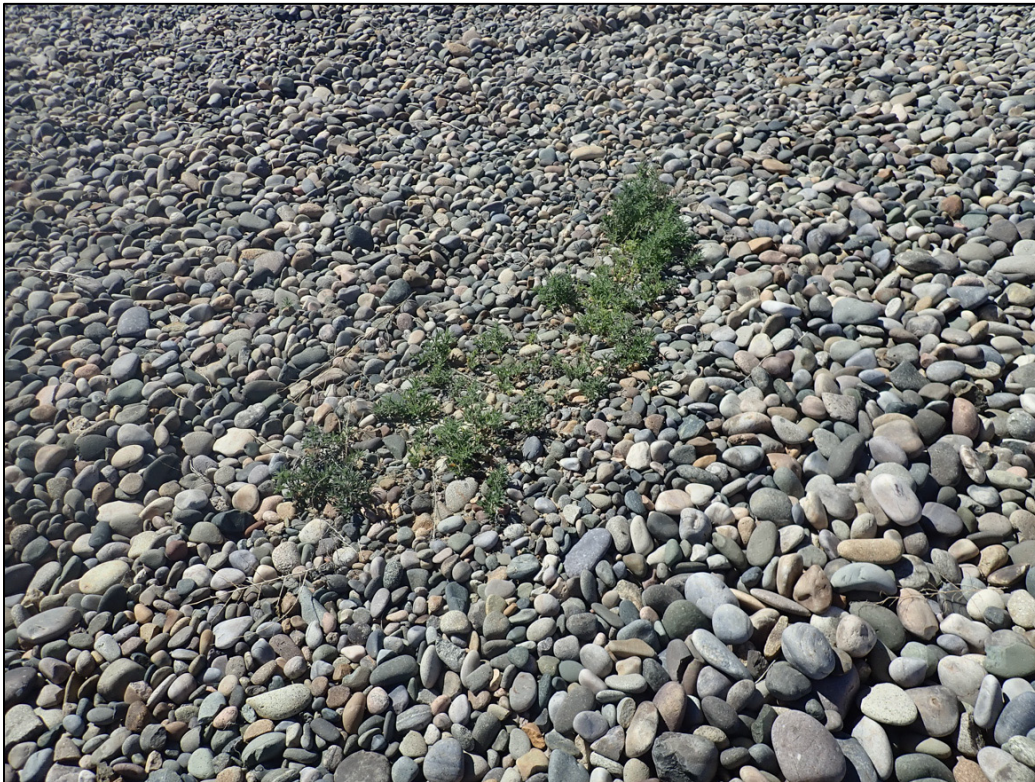
PL-4. Smaller Riprap Exposed Along Northern Ridge of Disposal Cell Top Slope
