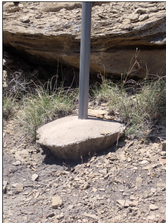
PL-2. Erosion Undercut at Concrete Base of Perimeter Sign P14
