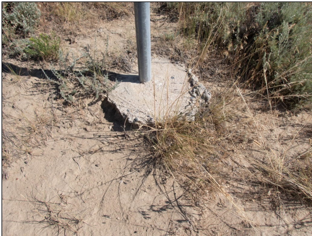
PL-2. Erosion Around Base of Perimeter Sign P3
