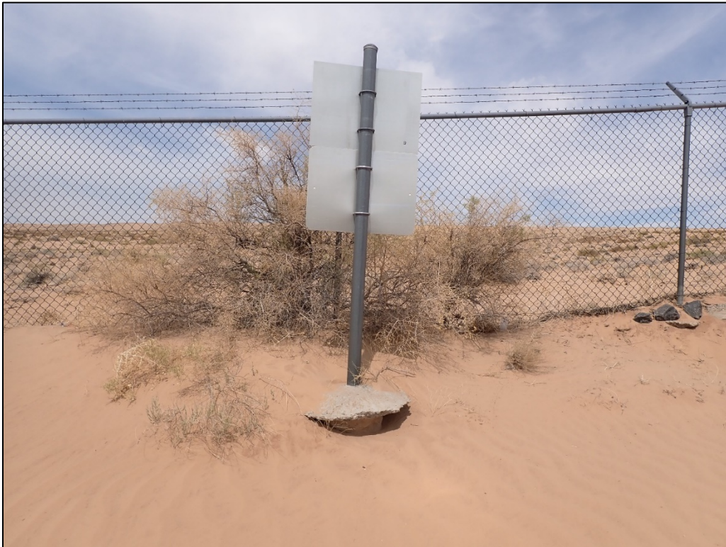
PL-5. Exposed Concrete Base of Perimeter Sign P9
