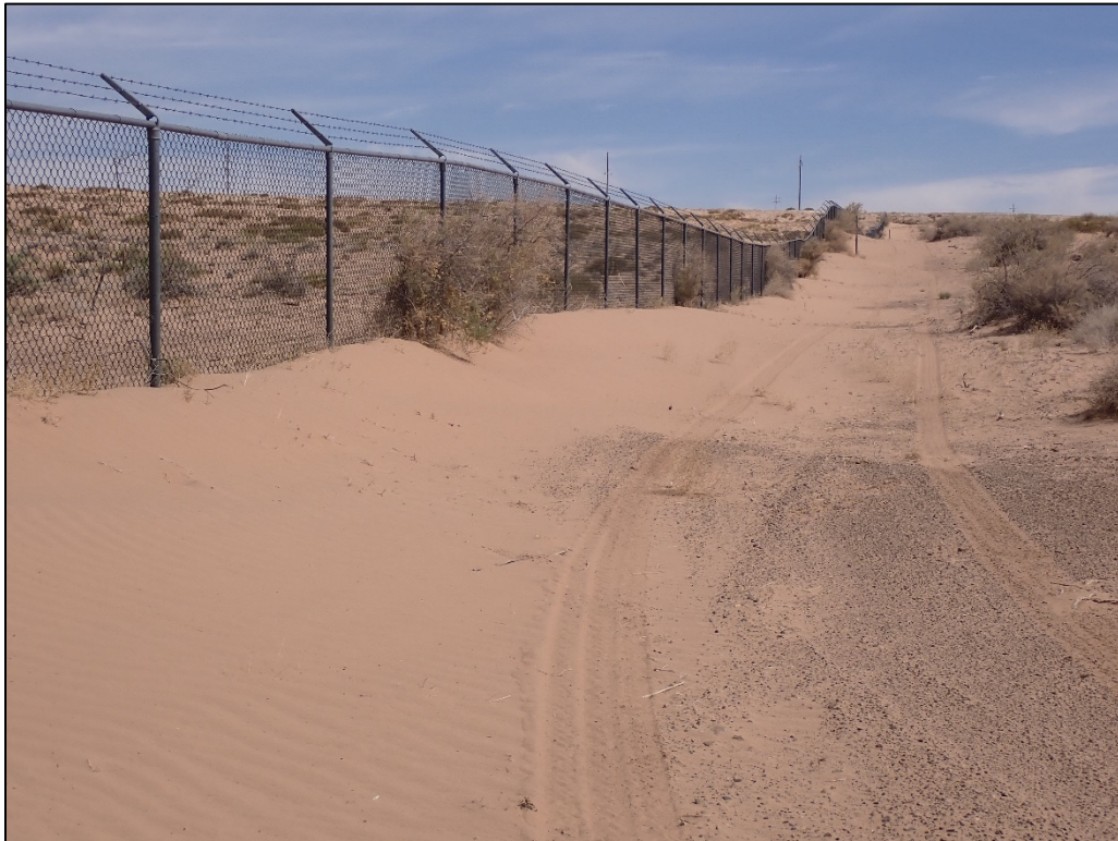
PL-1. Windblown Sand Accumulation Along Western Perimeter Fence
