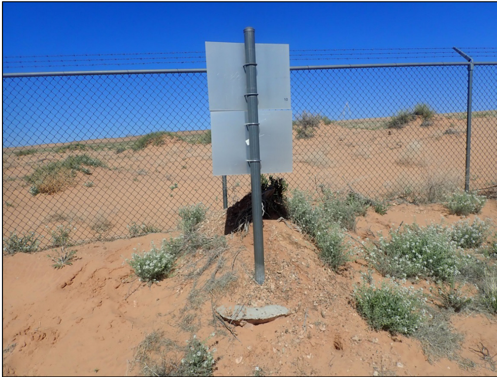
PL-5. Erosion Under Base of Perimeter Sign P10
