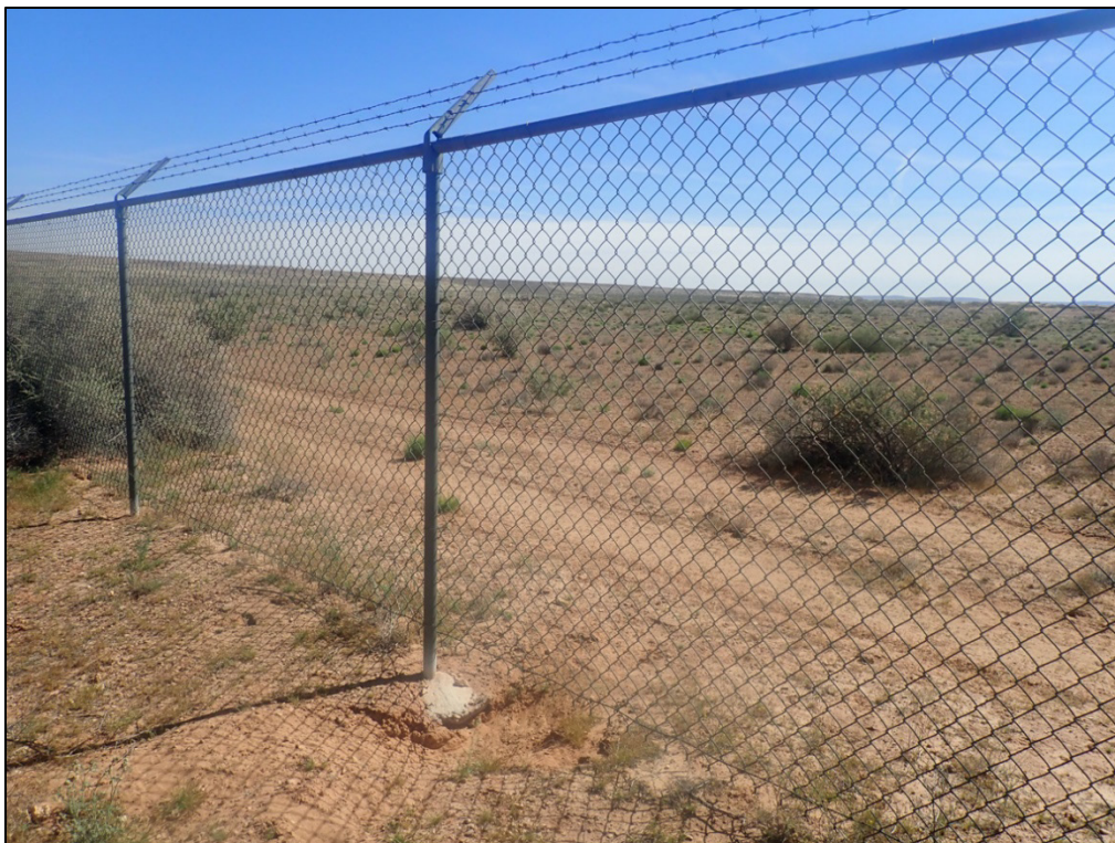
PL-2. Gap Created by Animals Under Fence Between Perimeter Signs P21 and P22
