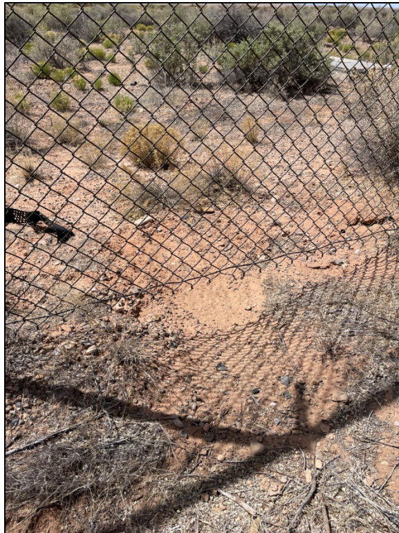
PL-2. Gap Created by Animals Under Fence Between Perimeter Signs P12 and P13
