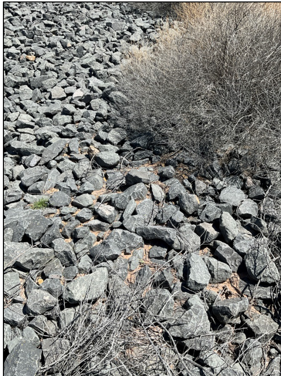
PL-10. Sediment Deposition on the South Slope of the Disposal Cell
