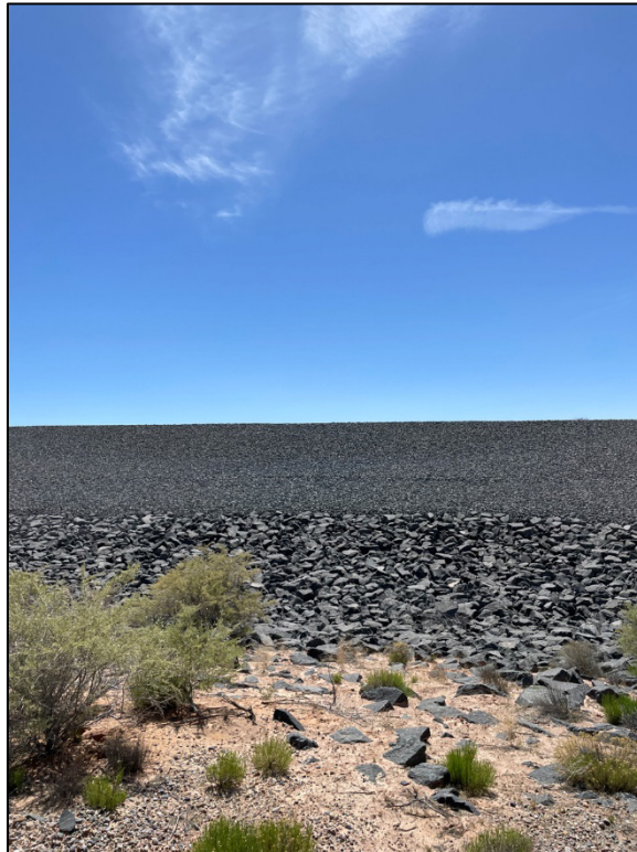
PL-9. Horizontal Lines on West Slope of Disposal Cell
