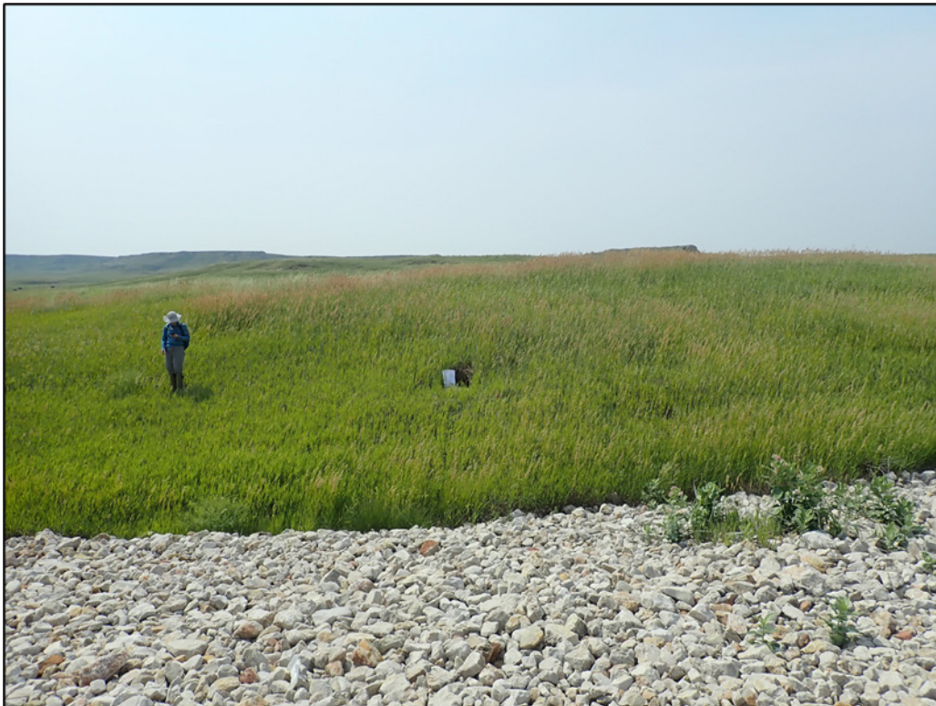
PL-8. Animal Burrow Adjacent to Toe of Armored Disposal Cell Side Slope
