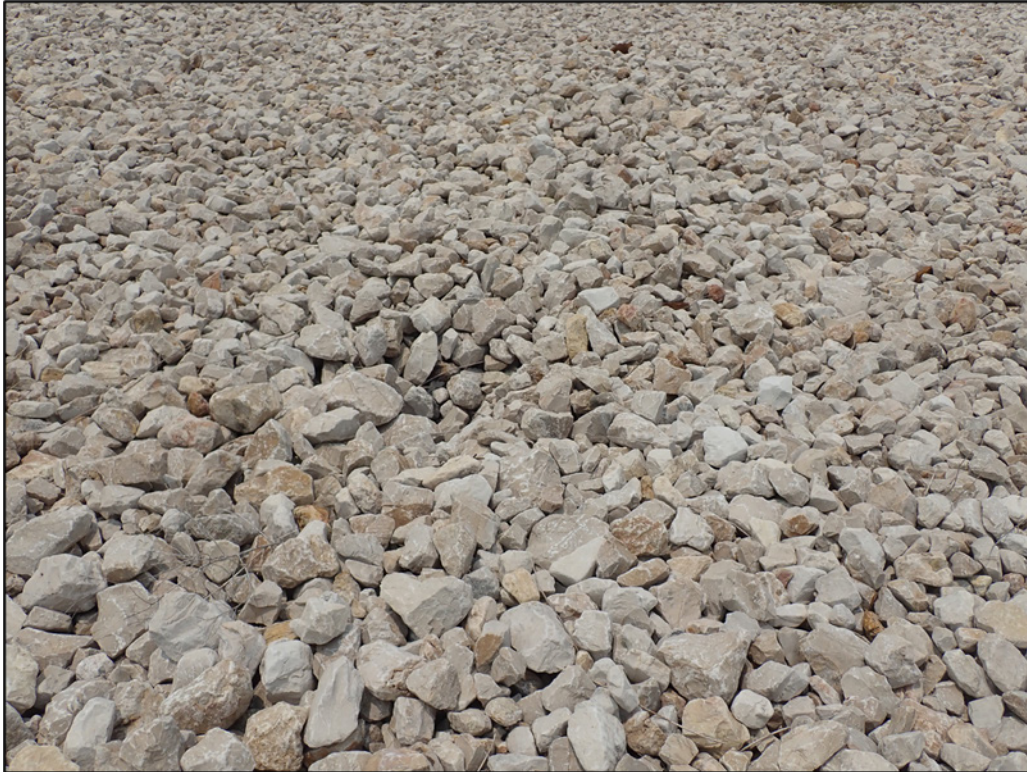
PL-7. Small Depression #2 on Disposal Cell Side Slope
