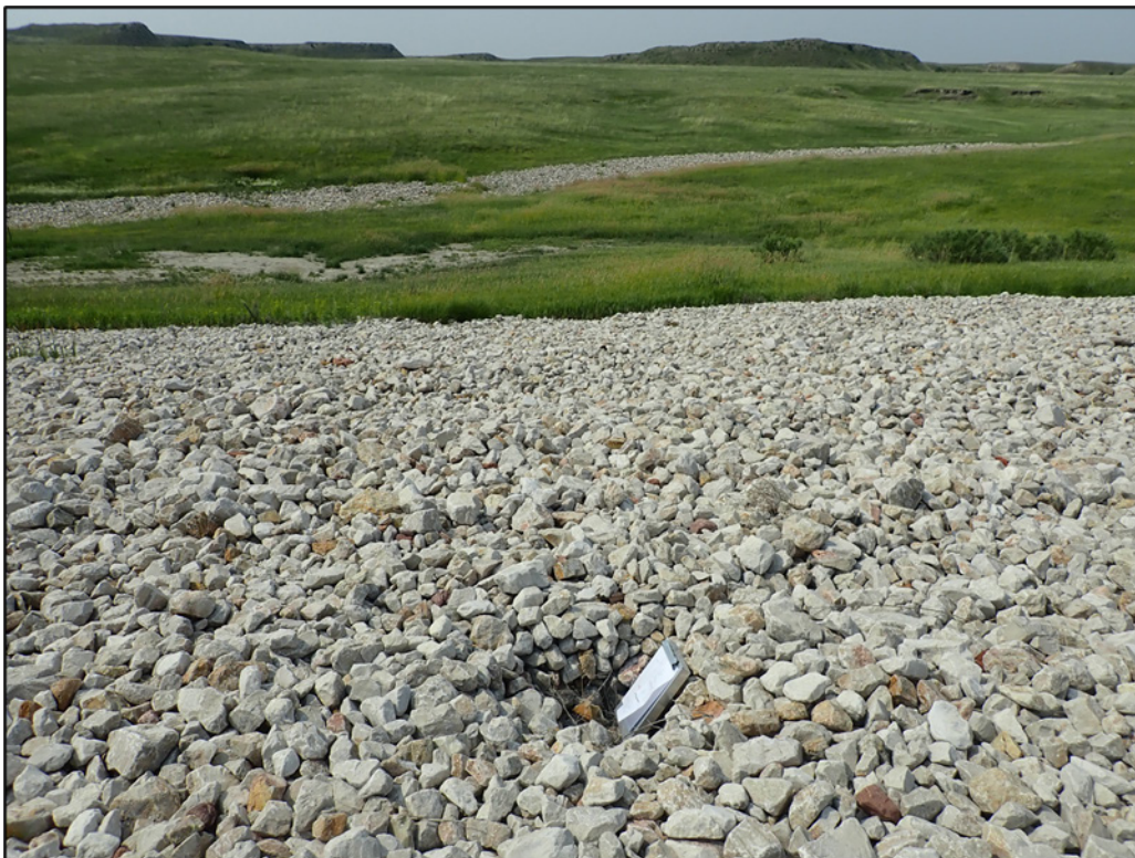
PL-6. Small Depression #1 on Disposal Cell Side Slope
