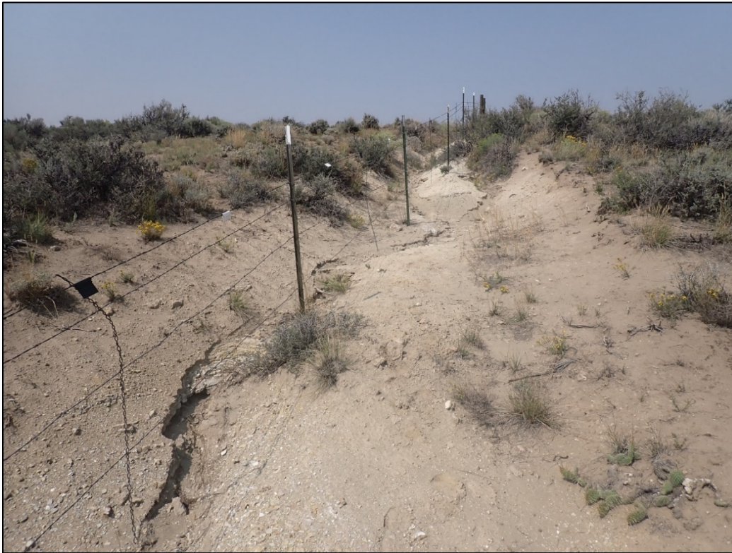
PL-1. Erosion Under the Perimeter Fence Southwest of the Disposal Cell
