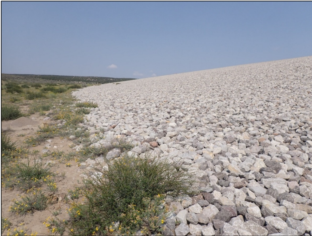
PL-11. Windblown Material Along Western Toe Slope of Disposal Cell
