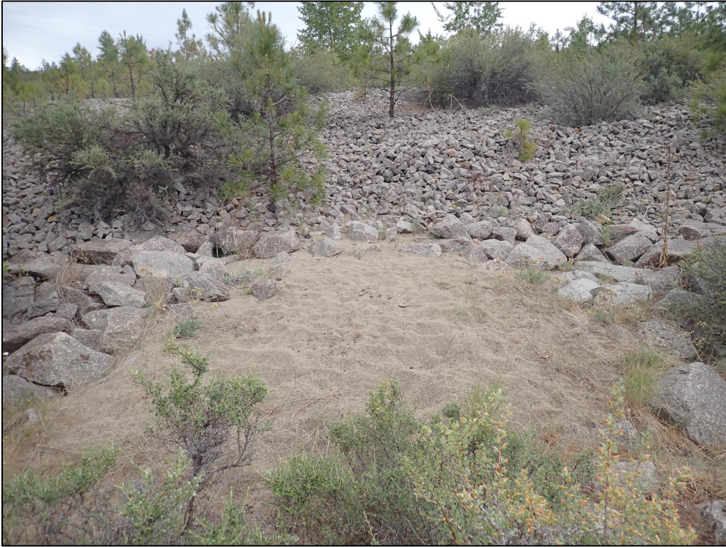
PL-11. Sand Deposit at Toe of Containment Dam Outslope
