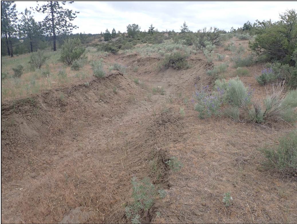
PL-6. Gully Downgradient of Riprap-Armored Swale Near Perimeter Sign P1
