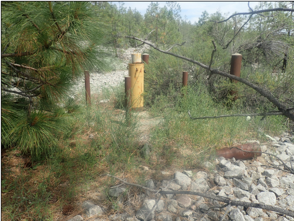
PL-4. Monitoring Well MW-4 with Damaged Bollard
