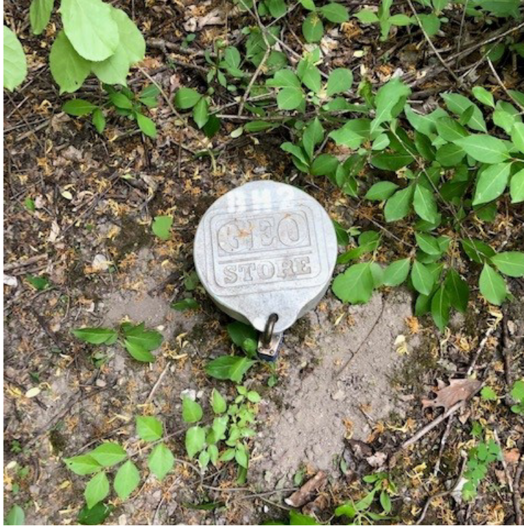
P01 - Monitoring Well BH2 at Plot M
