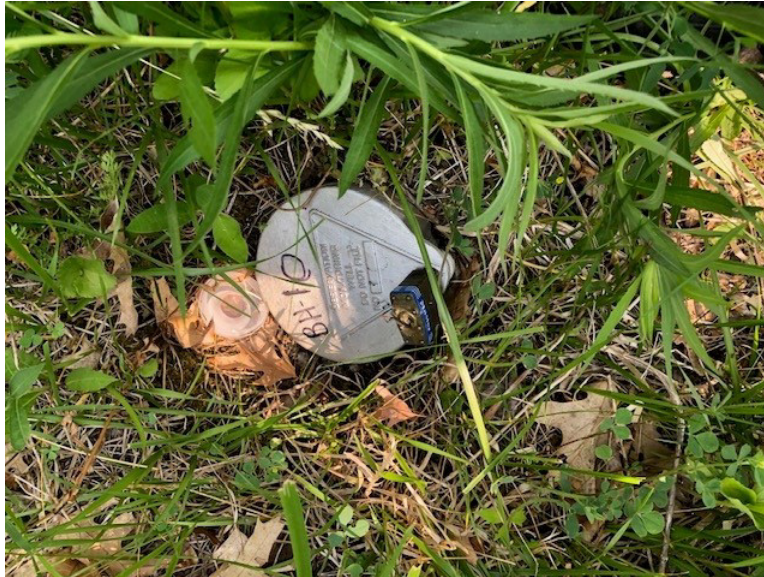
P05 - Monitoring Well BH10 at Plot M
