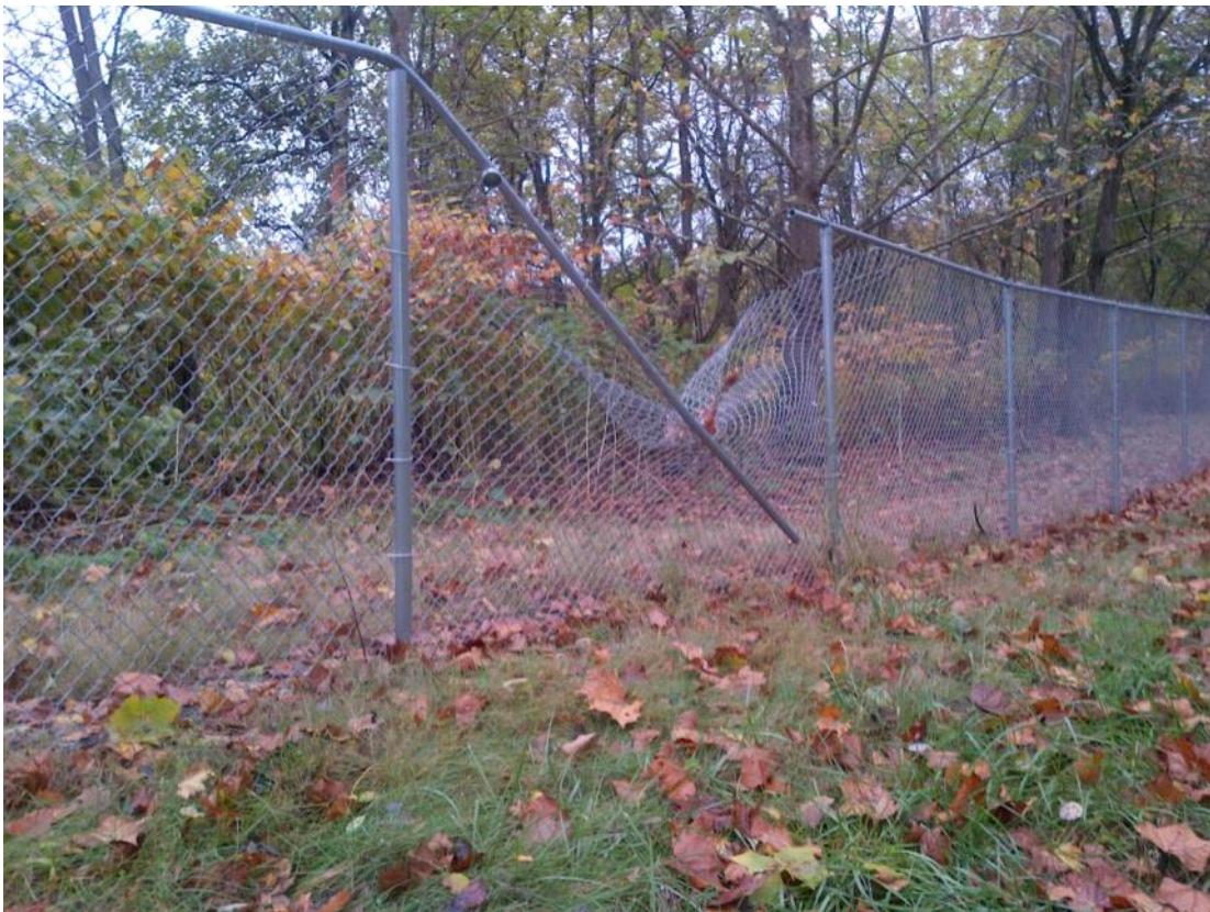
BUR 10/2014. PL-2. Damage to perimeter fence.
