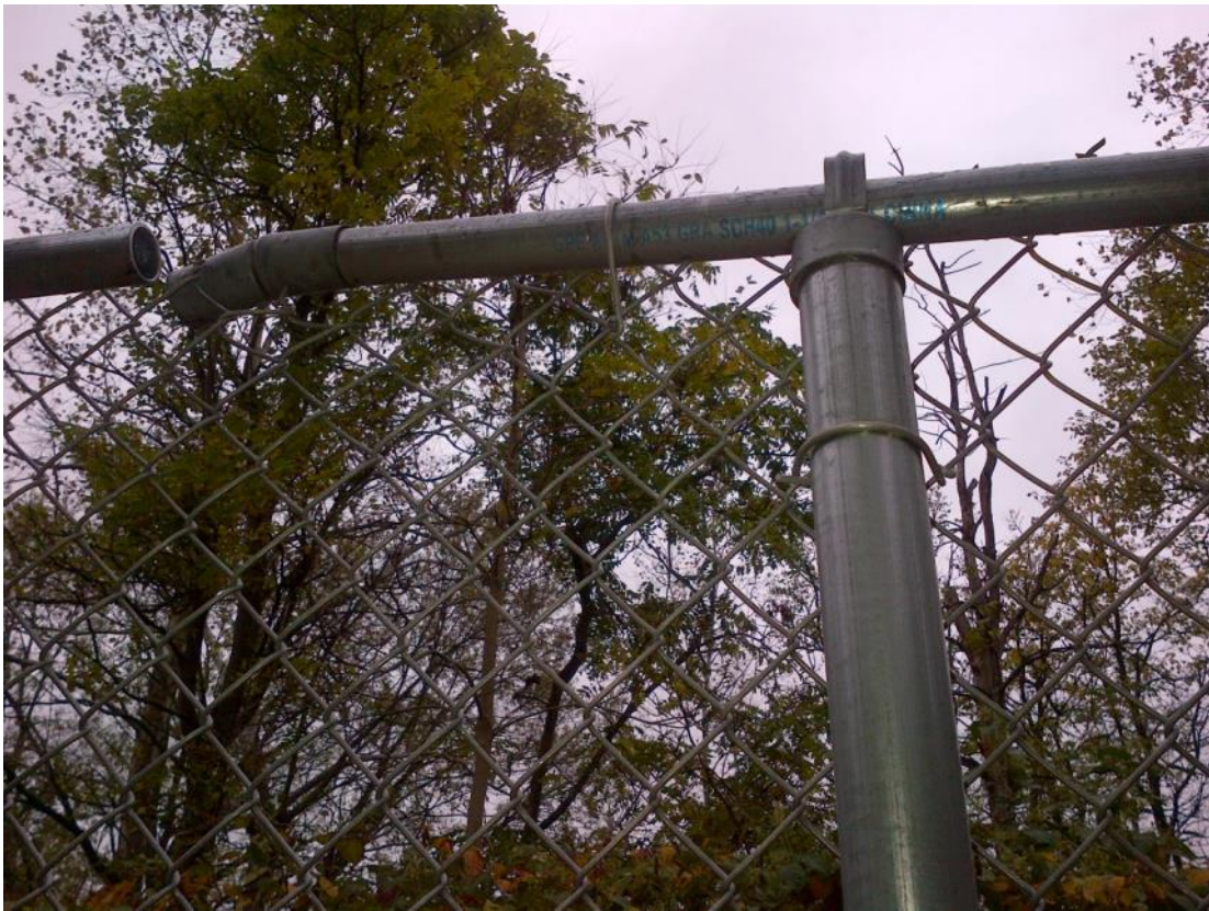
BUR 10/2014. PL-3. Damage to top rail of perimeter fence.
