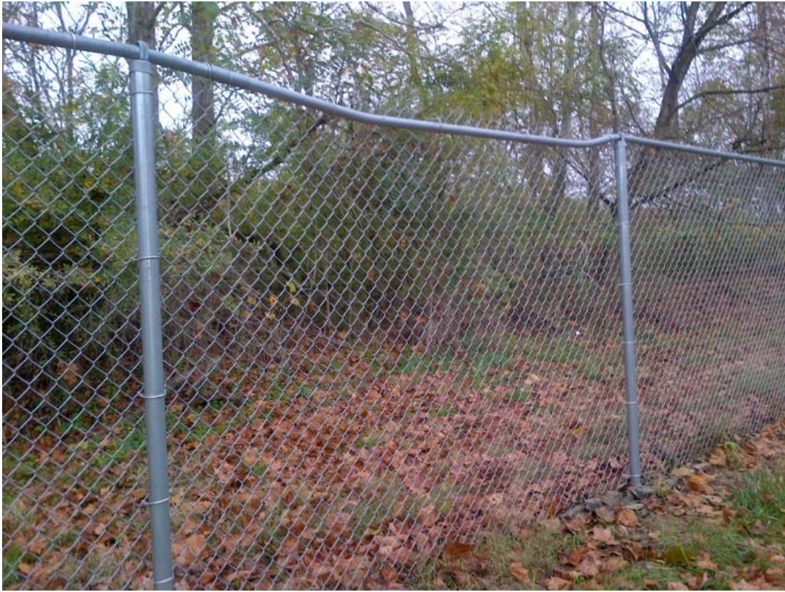
BUR 10/2014. PL-1. Slight damage to top rail of perimeter fence.
