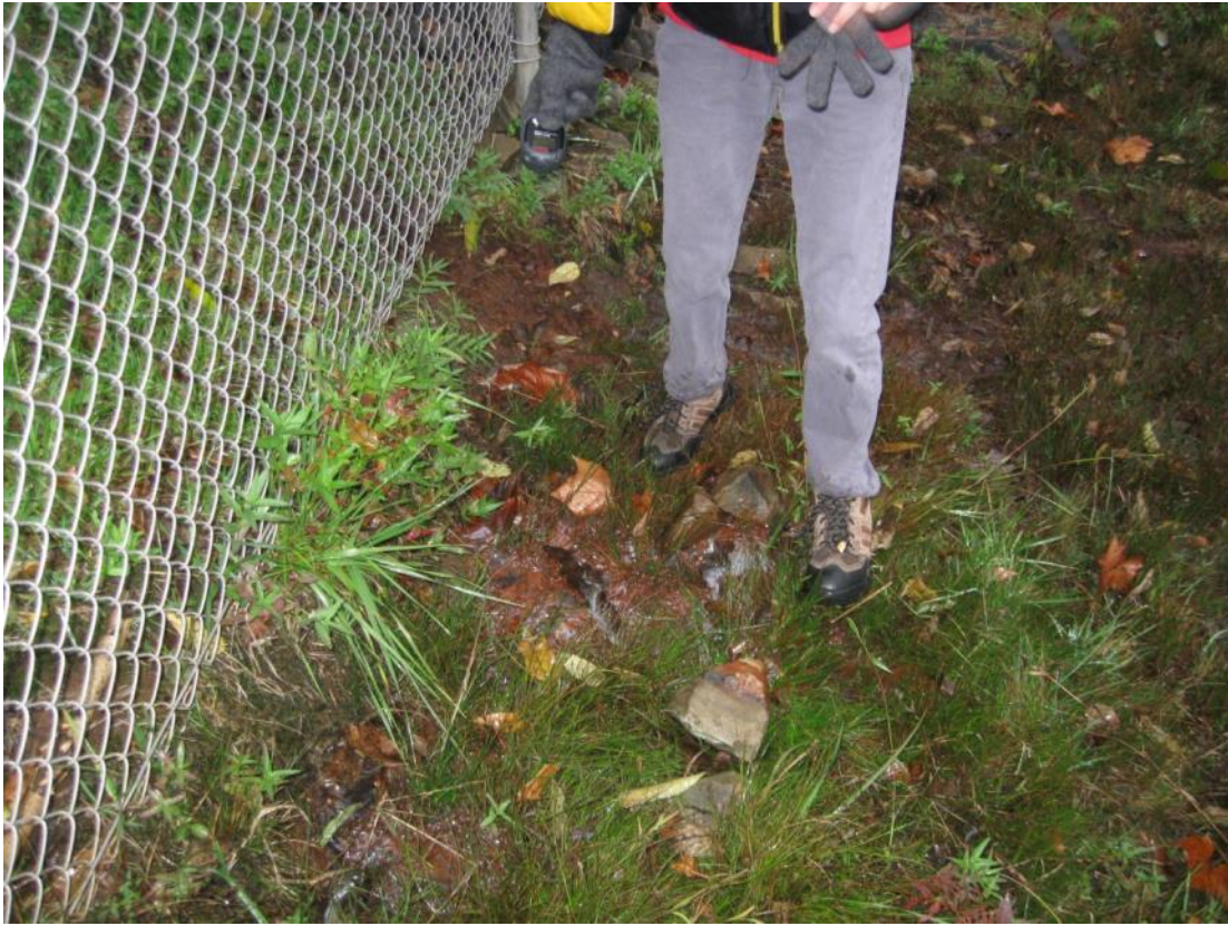
BUR 10/2014. PL-15. Active seep northwest of disposal cell.
