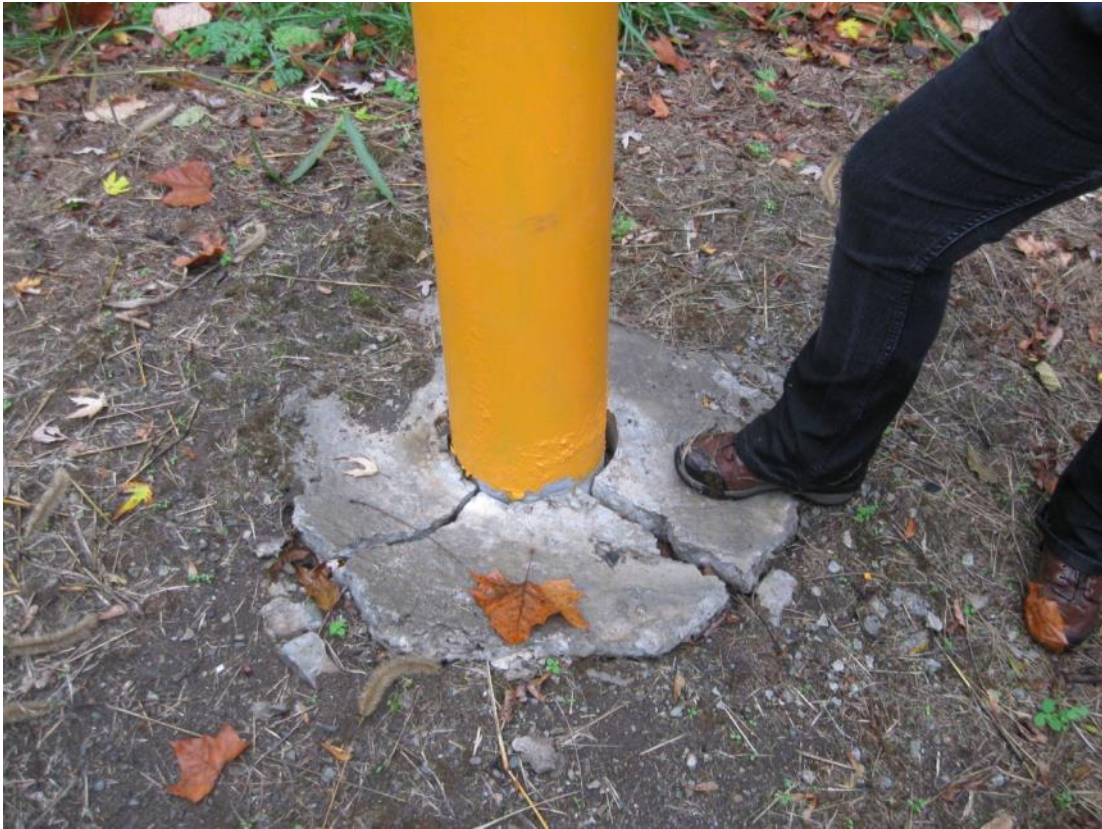
BUR 10/2014. PL-9. Broken concrete around base of monitoring well 0523.
