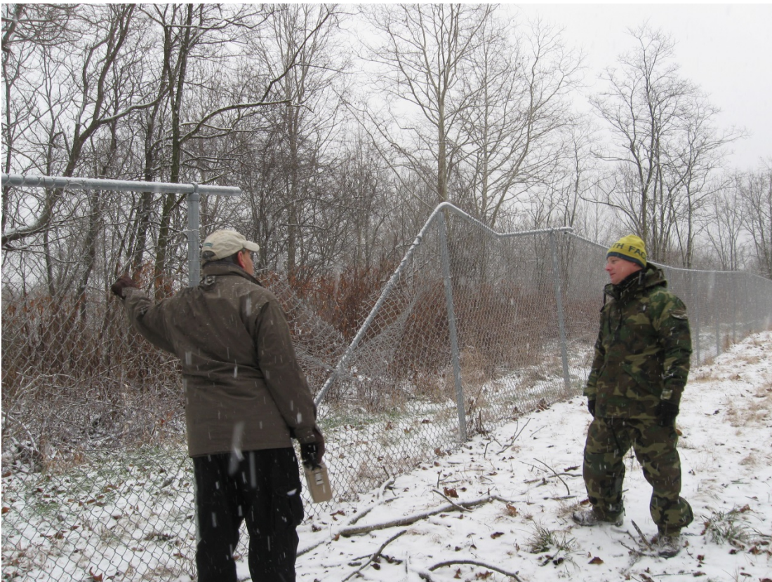
BUR 12/2013. PL-5. Damaged fence east of perimeter sign P11.
