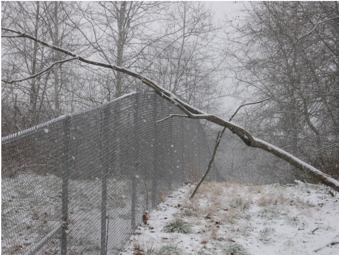
BUR 12/2013. PL-2. Tree down on south fence.
