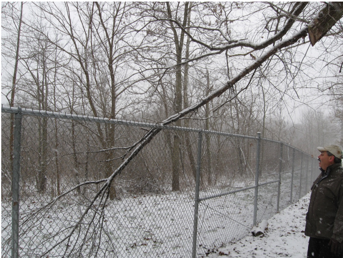
BUR 12/2013. PL-3. Tree across southern fence.
