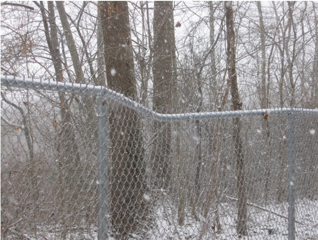
BUR 12/2013. PL-4. Damaged fence east of perimeter sign P12.
