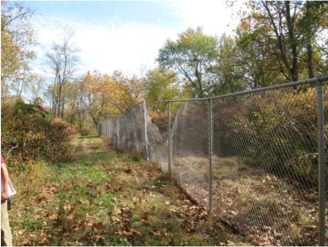
BUR 10/2012. PL-1. Fence damage.
