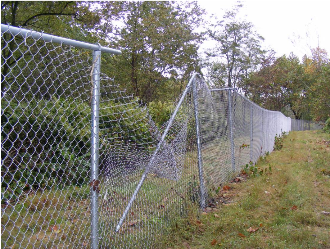
BUR 10/2011. PL-1. Damage to perimeter fence.
