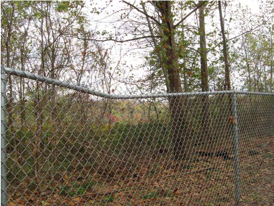
BUR 10/2010. PL-1. Bent rail on top of south perimeter fence.
