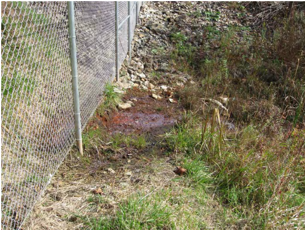
BUR 10/2009. PL-6. Active seep under the north perimeter fence.
