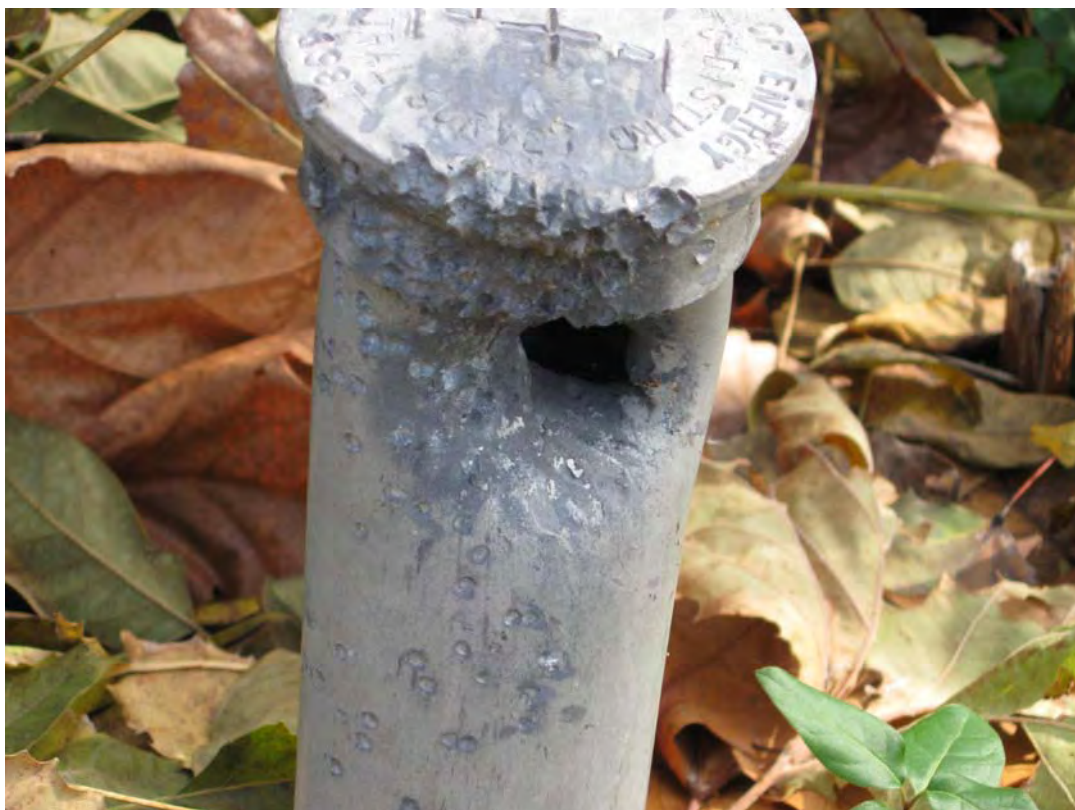
BUR 10/2009. PL-2. Erosion control marker E-7 damage, possibly by grass-cutting equipment.
