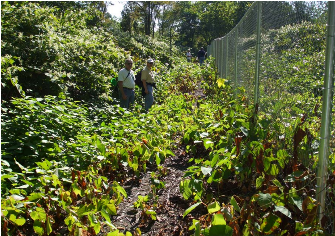
BUR 9/2007. PL-2. Vegetation encroaching on new fence.
