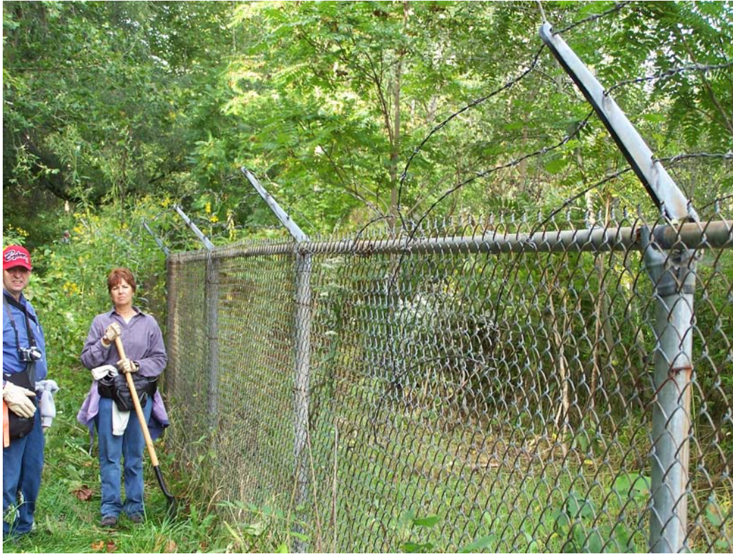
BUR 9/2006. PL-1. Broken strands of barbed wire on south fence line.
