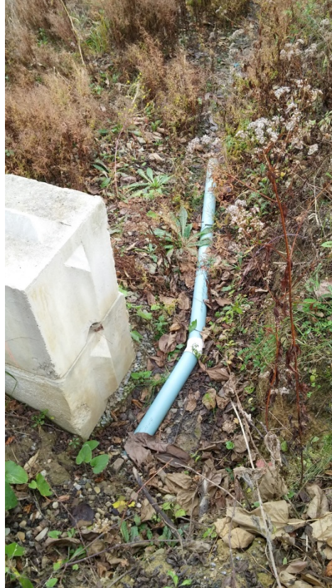
CAN 10/2015. PL-3. Drainage pipe from storage building, next to monitoring well MW-0414B.
