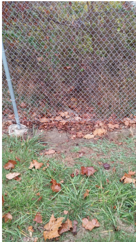
CAN 10/2015. PL-6. Gap beneath fence fabric and ground in area of erosion.
