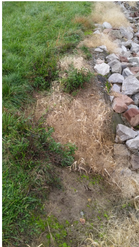
CAN 10/2015. PL-14. Small area of erosion along the bank of Chartiers Creek, above armored riprap.
