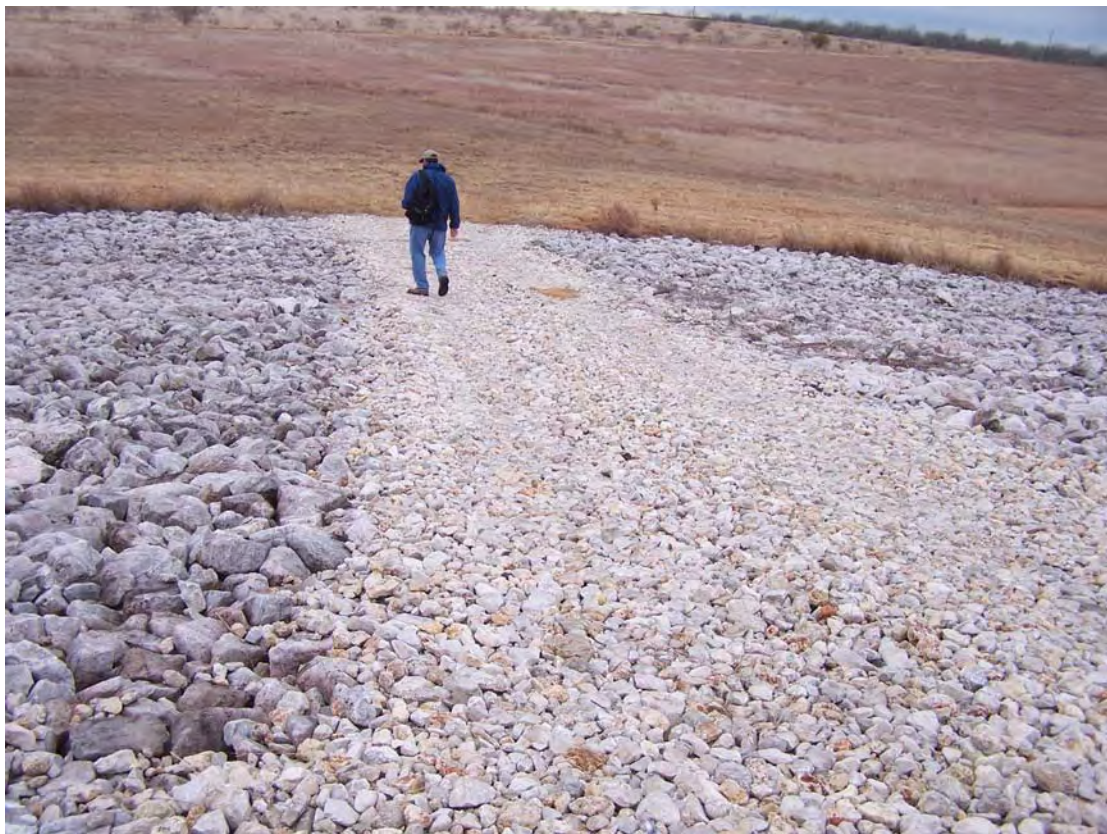
FCT 1/2008. PL-4. Aggregate ramp on the west corner of the disposal cell.
