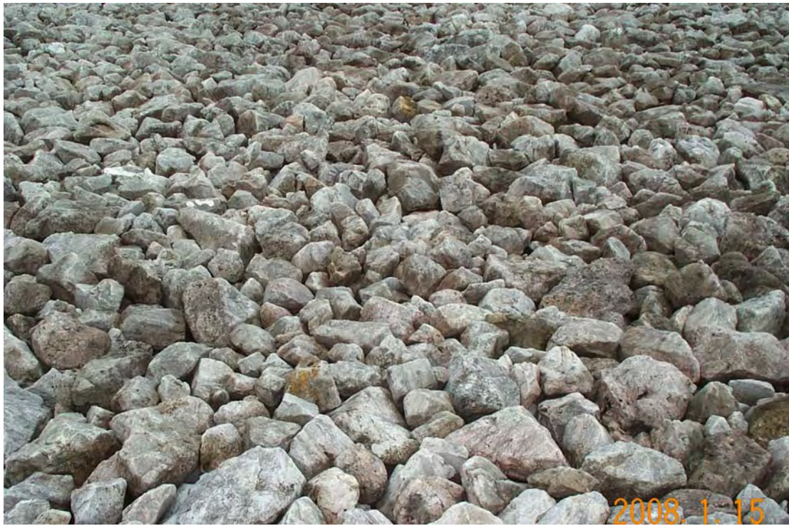
FCT 1/2008. PL-3. Reference photo of riprap adjacent to disposal cell access ramp.
