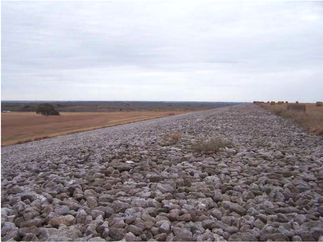
FCT 1/2008. PL-1. Northwest side slope of the disposal cell; hay bales on cell top.
