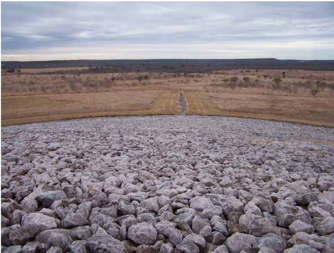
FCT 1/2008. PL-6. South side slope of the disposal cell; south rock drain in the background.
