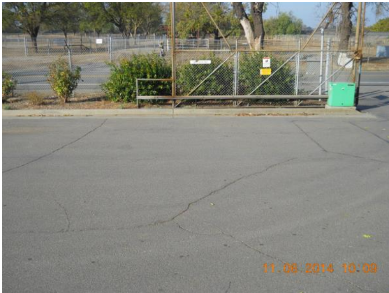
View west over Dry Wells A-E Area: site entrance gate and Old Davis Road in background.
