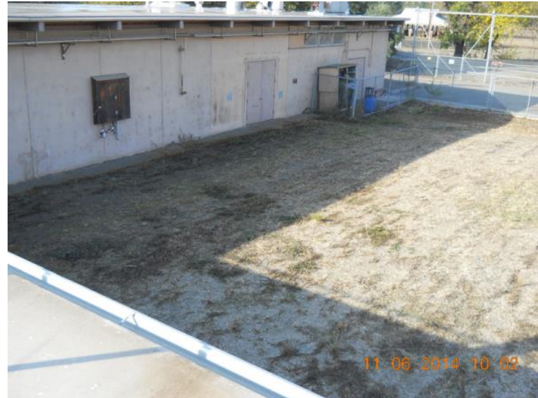
Roof-level view southwest over Domestic Septic System 2 area within middle portion of Radium/Strontium Treatment Systems Area: Building H-218 in background.
