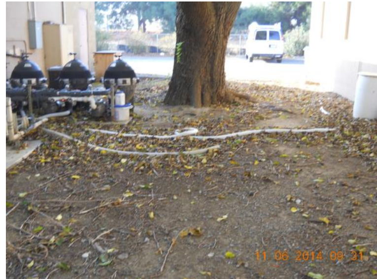
View south over septic tank part of Domestic Septic System 3 Area: Building H-216 to left; Building H-215 to right.
