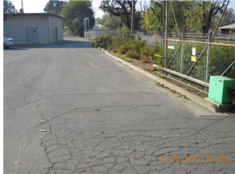
View south over Dry Wells A-E Area: Building H-219 in background/left; facility entrance in the lower right-hand corner.
