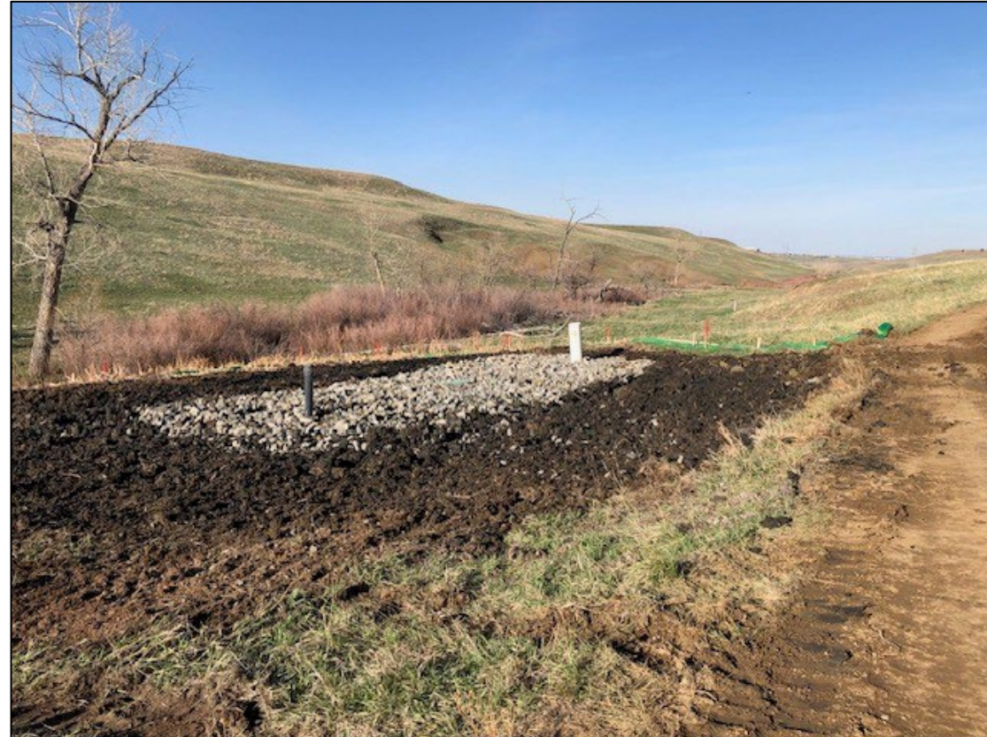
SPPTS discharge gallery
