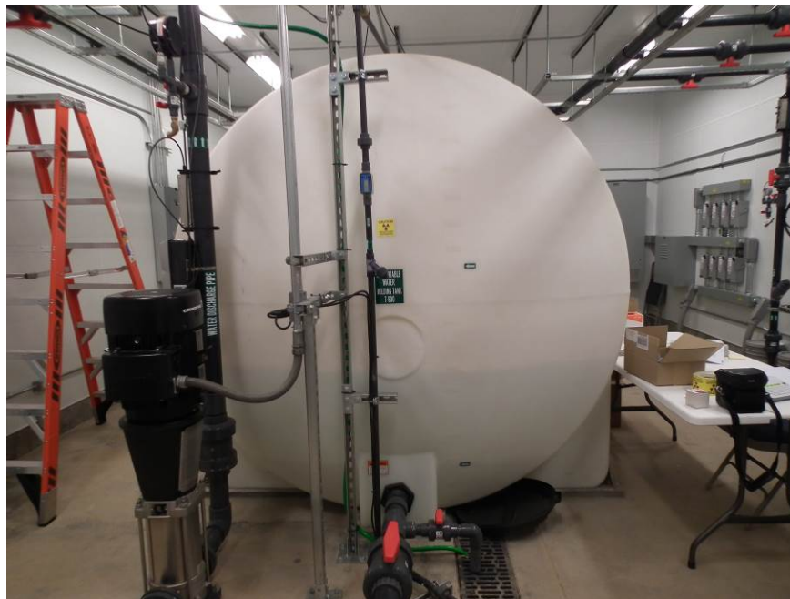
Figure 5. Photograph of Interior of GTB Showing Groundwater Transfer Tank
