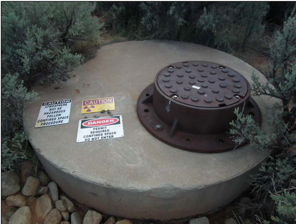
PL-18. Manhole 5 Showing Current Postings
