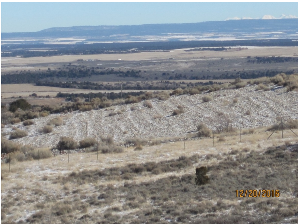
Figure No. 2, Horizontal ridges on a Northwest riprap slope, Monticello, UT, [from 2016 & 2017 report]
