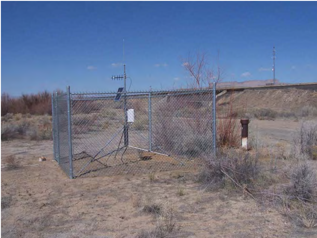
GRN 3/208. PL-4. Telemetry tower and enclosure at well MW-0817.
