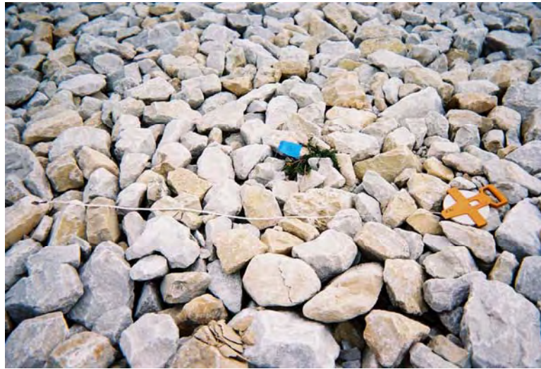
Photo 7. Cell cover rock test plot TP4; located on upper west side (2003 Inspection).
