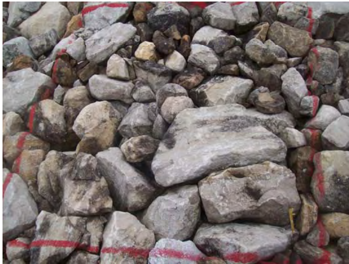
Photo 2. Cell cover rock test plot TP1; north edge of north facet (2009 Inspection).
