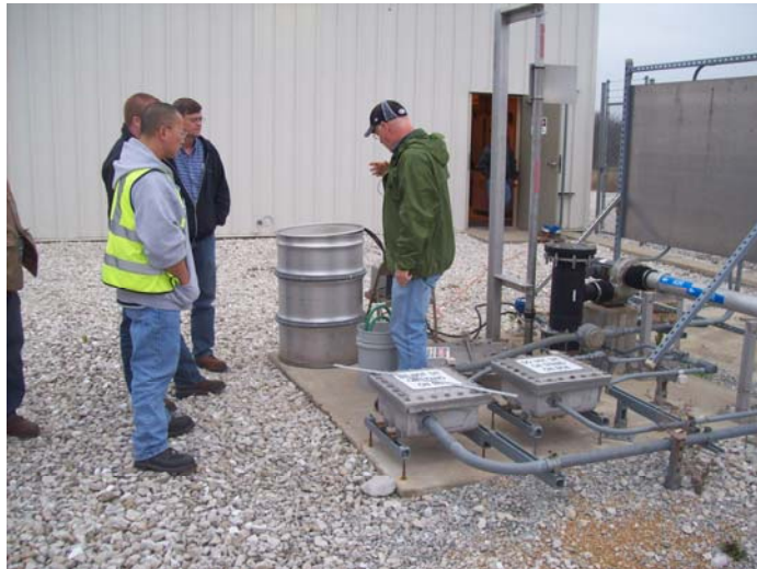
Photo 20. Sump outside LCRS Building.
