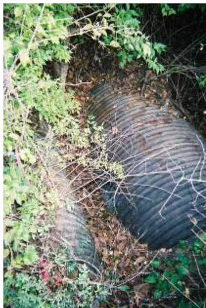
Photo 12: Eroded area where culverts are exposed in ditch between Highway D and outlet end.
