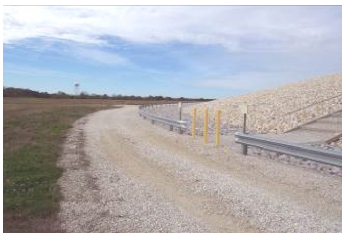
Photo 24: Guard rail around disposal cell.
