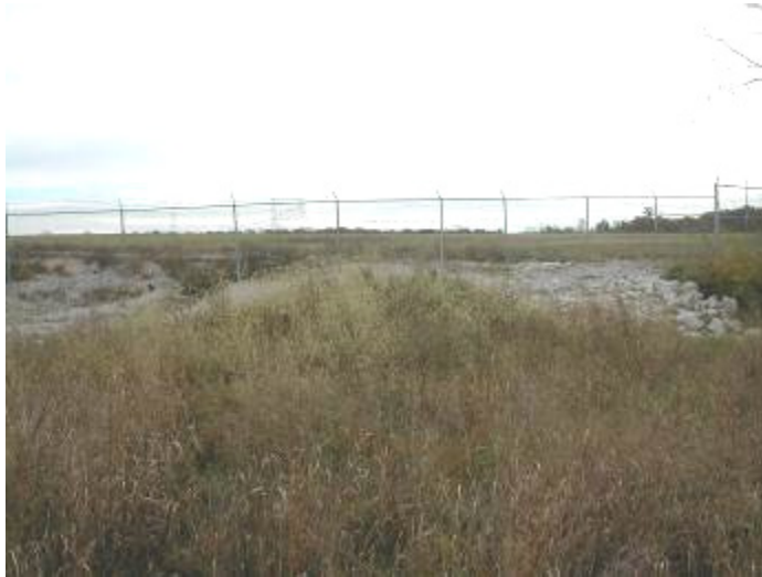
Photo 28: Area of erosion onto the Army property. The eroded ditch is to the left and outfall NP-0050 is to the right.
