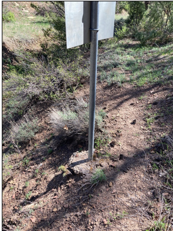
PL-5. Perimeter Sign P56 with Undercut Base and Unstable
