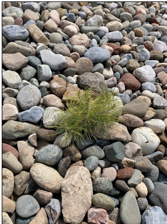
PL-10. Woody Plant Growing in Riprap
