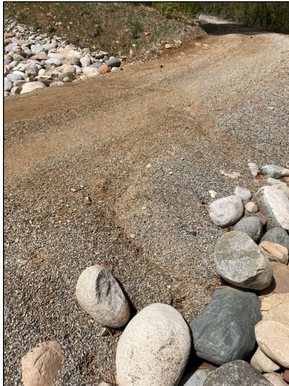
PL-1. Access Road Erosion
