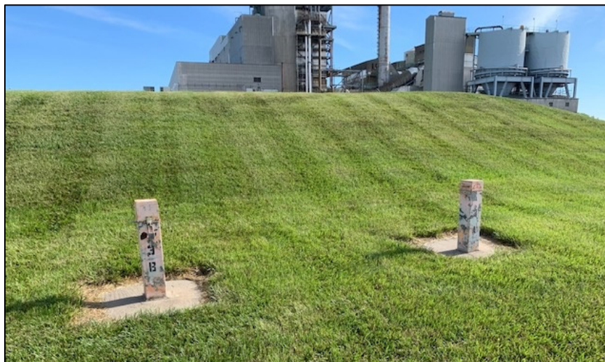
Photo 5. Condition of Outer Casing of Monitoring Wells
