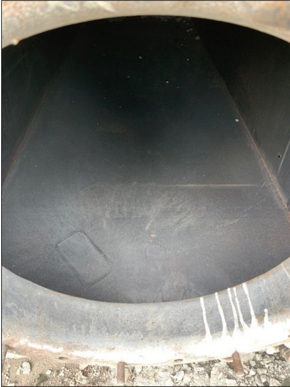
Figure 7. Room B-7 Tank, Internals
