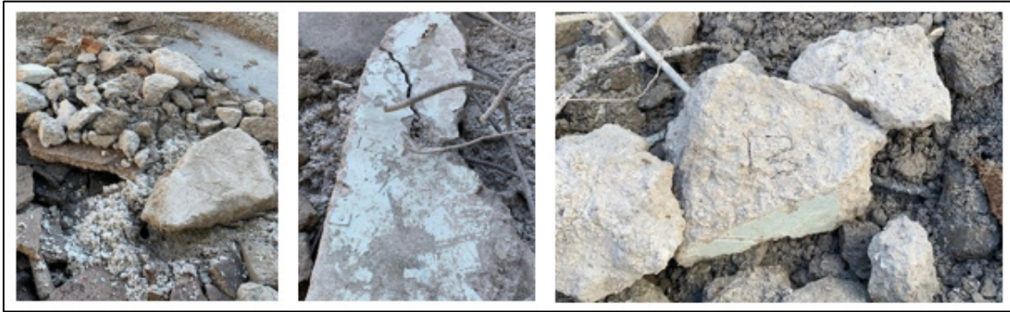
Figure 4. Rubblized Wall Concrete
