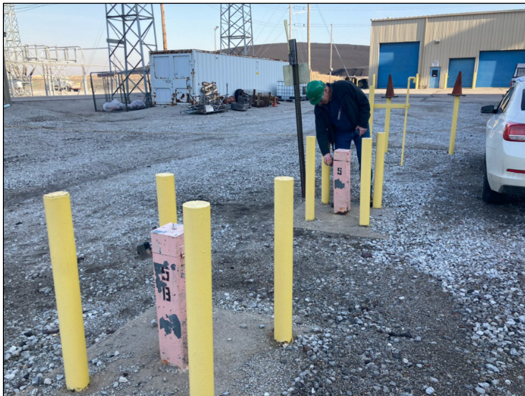
Photo 6. Example of Monitoring Wells' Outer Casing Requiring Repainting
