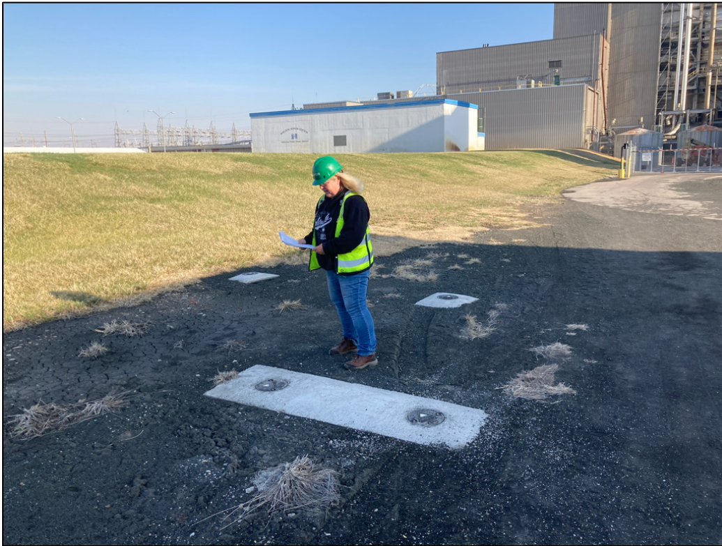
Photo 4. Flush-Mount Monitoring Wells OBS-2A, OBS-2B, OBS-2B2, and OBS-2C2
