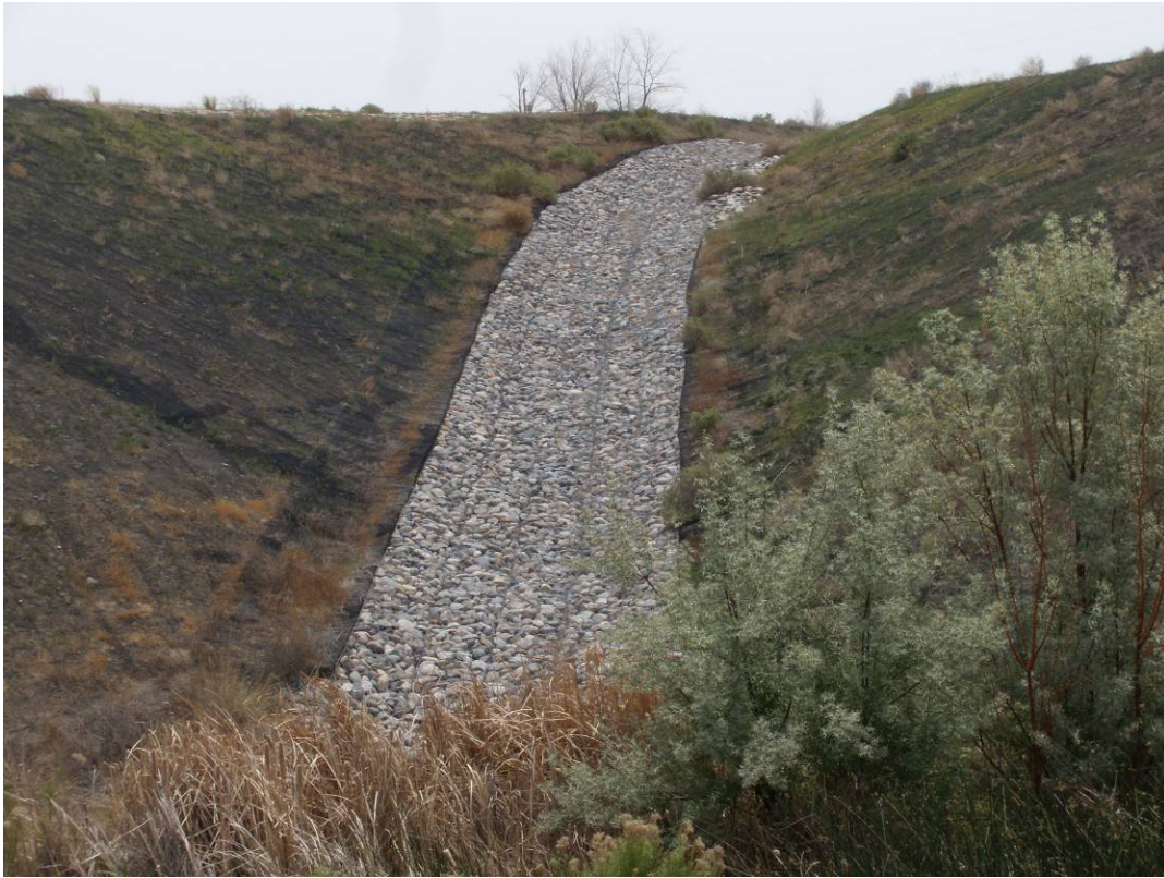
SHP 6/2011. PL-3. Outflow channel.
