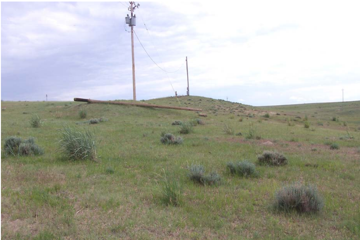
SPK 6/2007. PL-2. New utility pole with transformers; new power pole for the onsite water supply well in background.
